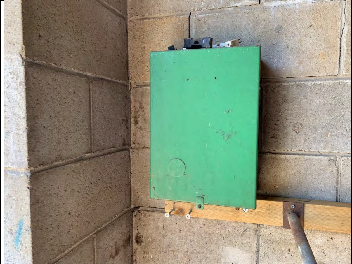
Photo 42 – View of the fuse box in Garage #2.
