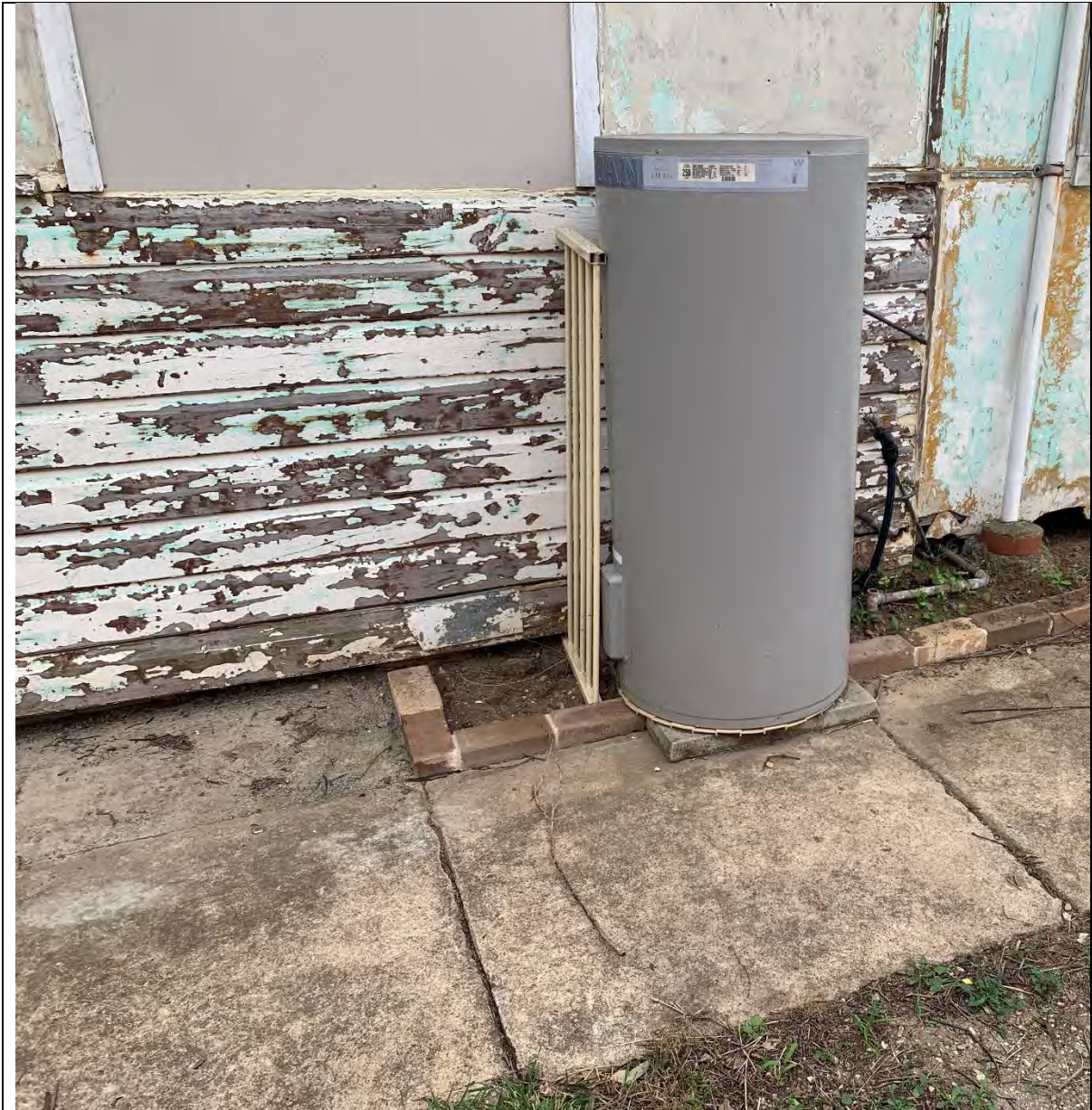
Photo 43 – View of the water heater located on the south side of the residence. The water heater could contain SMF.
