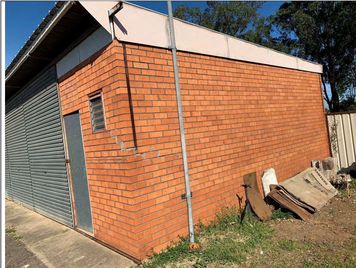
Photo 30 - View to the southwest showing Garage #1. The fascia trim at the top of the northern wall is composed of non-friable asbestos cement sheet cladding. Identical non-friable asbestos cement sheeting is located on the east side of the garage.
