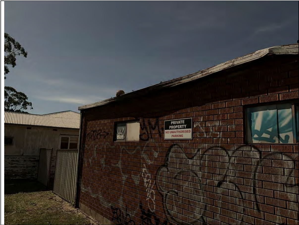
Photo 32 - View to the north showing the southern side of garage #1. The fascia wood trim is covered with brown lead-based paint.
