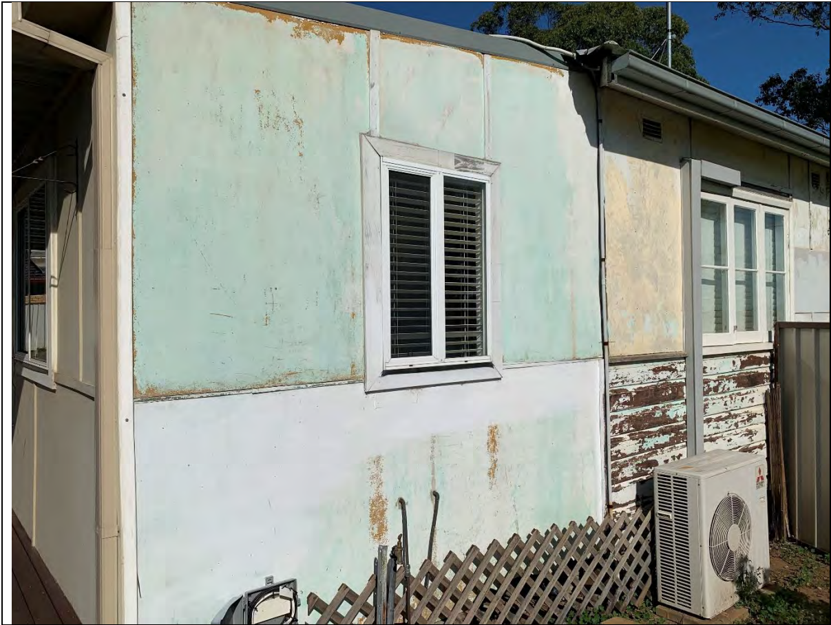
Photo 11 - View to the south showing the northeast corner of the residence. The wall in the immediate foreground is composed of non-friable asbestos cement sheet cladding. The wall further to the west is composed of wood cladding covered with lead-based paint on the lower portion of the wall and asbestos cement sheet cladding covered with lead-based paint on the upper portion of the wall.
