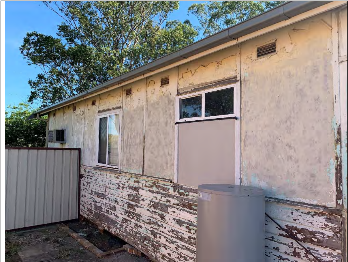
Photo 4 - View to the west showing wood cladding covered with white flaking lead-based paint on the lower portion of the wall. The upper portion of the wall consists of non-friable asbestos cement sheeting covered with white and aqua coloured lead-based paint.
