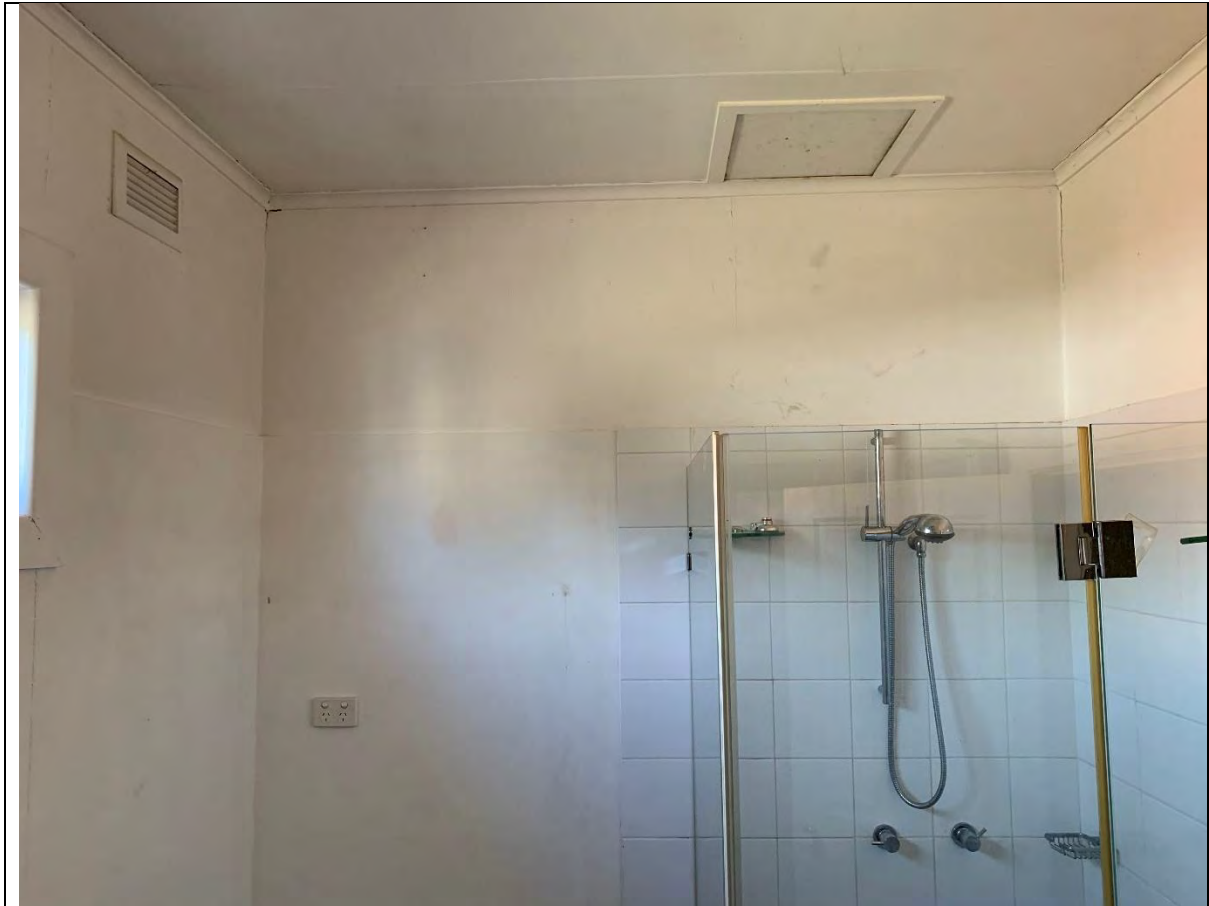
Photo 19 - View to the west showing the bathroom. The ceiling and the wall (partially covered by particle board) is composed of non-friable asbestos cement sheeting covered with lead-based paint.
