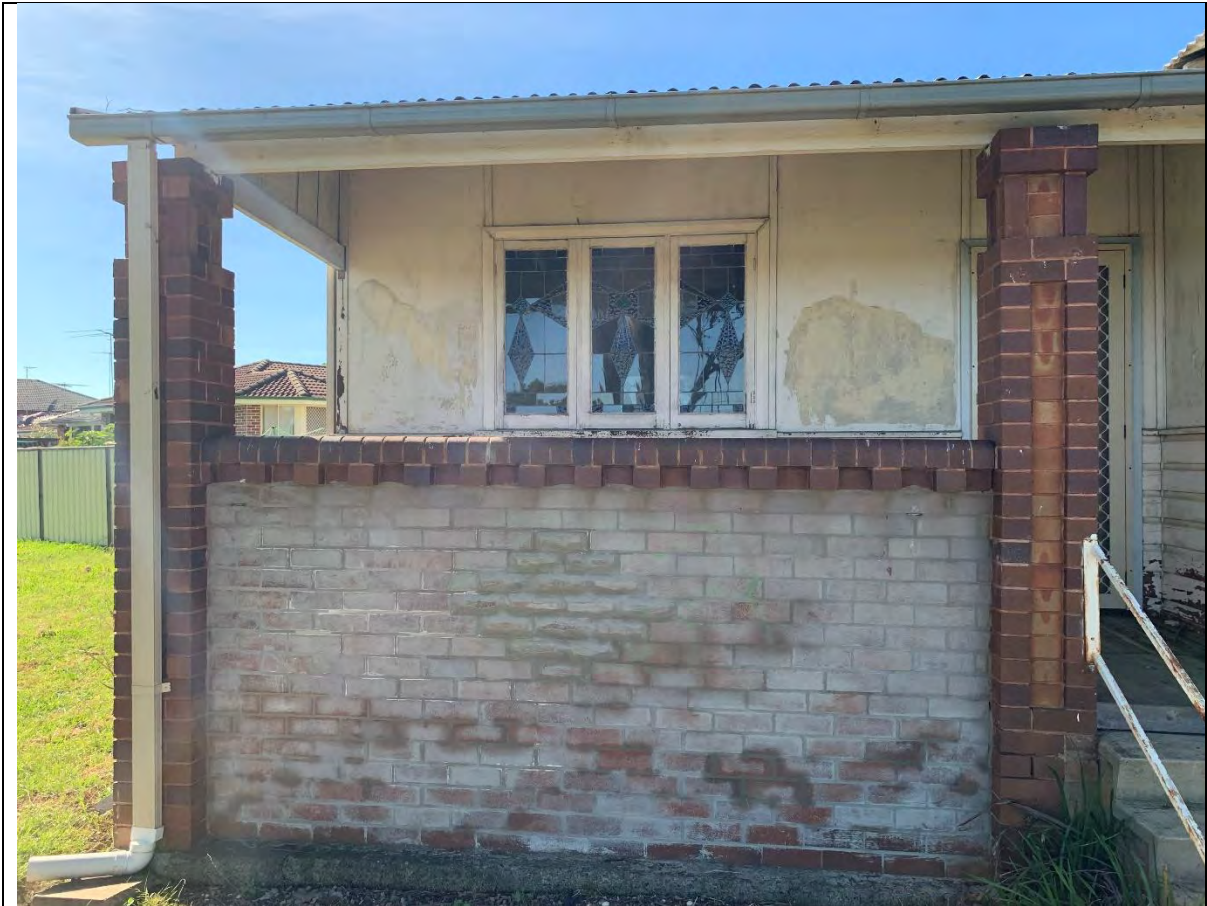
Photo 7 - View to the east showing the patio on the west side of the house. A stained-glass window is shown. The comes in the window (parts holding glass together) are presumably composed of lead.
