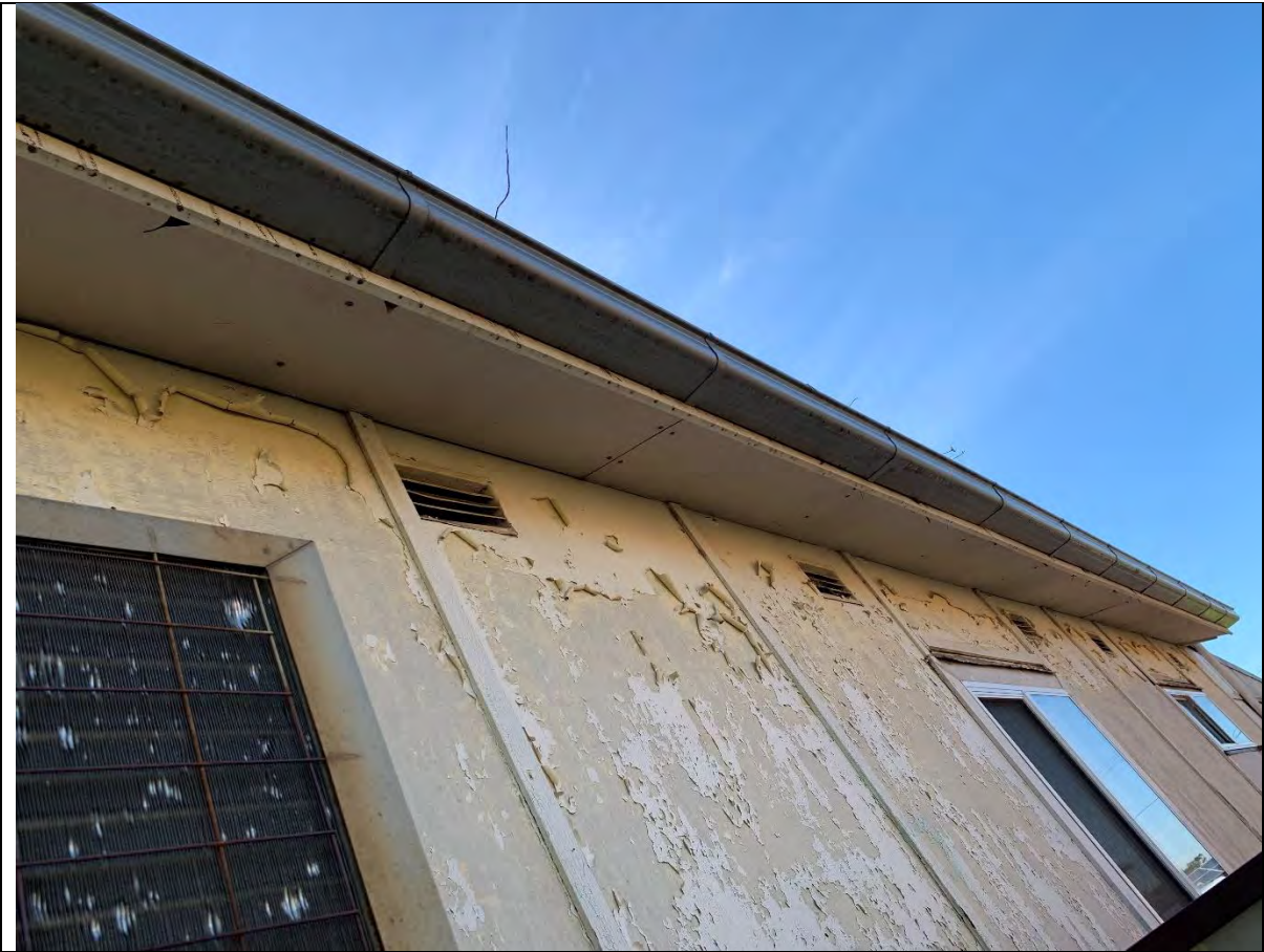
Photo 5 - View of the soffit underlying the eaves on the east (south) portion of the residence. Also shown is the non-friable asbestos cement sheet cladding covered with white and aqua lead-based paint.
