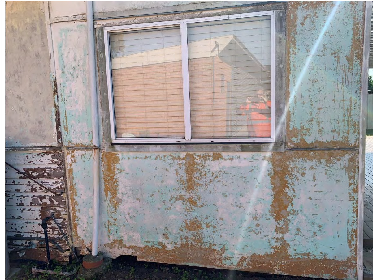
Photo 2 - View to the north showing non-friable asbestos cement sheet cladding covered with flaking lead-based paint. Sheeting with missing sections can be observed in the lower left-hand corner.
