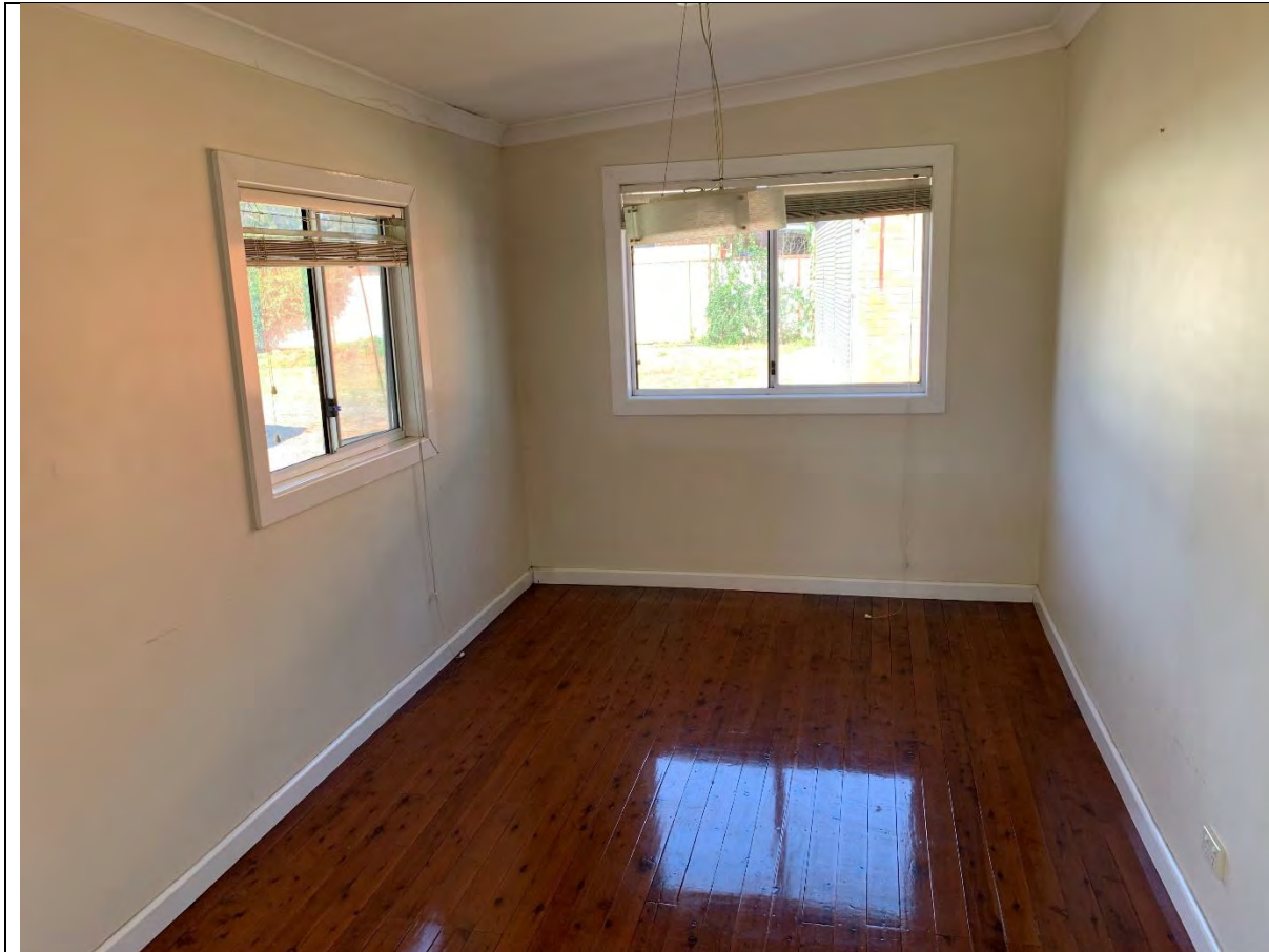
Photo 16 - View to the south showing the living room (Room 1). The walls and ceiling are covered with lead-based paint. The floor is composed of wood. The walls and ceiling are composed of gyprock.
