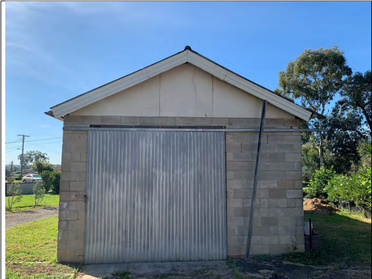
Photo 36 - View looking to the east showing Garage #2. The roof is covered with non-friable asbestos cement corrugated roofing material. The gable is clad with asbestos cement sheet cladding.
