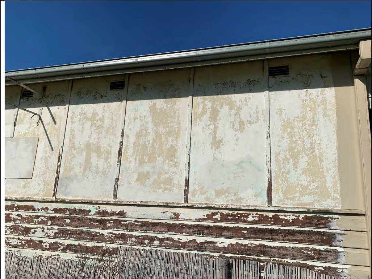
Photo 10 - View towards the south showing the north side of the residence. Wood cladding covered with lead-based paint is present on the lower portion of the wall and non-friable asbestos cement sheet cladding covered with lead-based paint is present on the upper portion of the wall.
