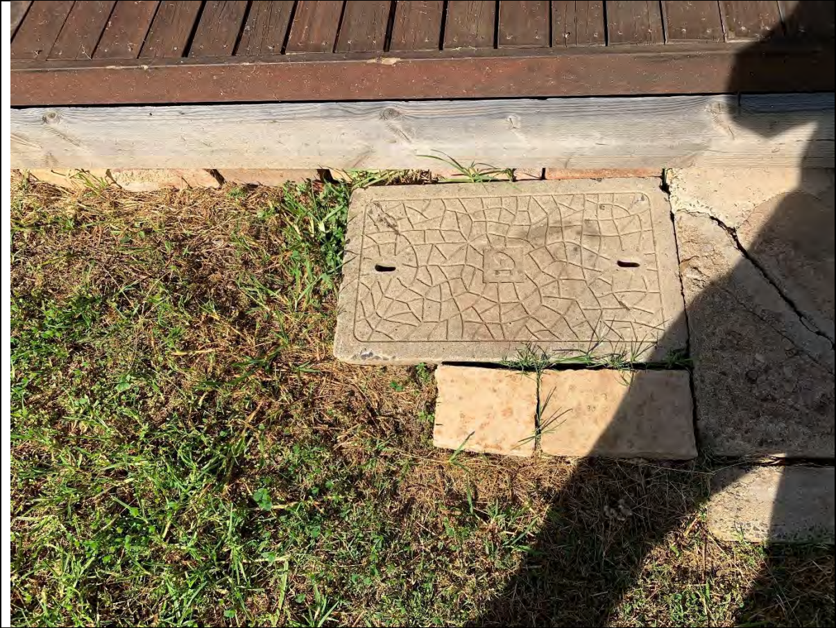
Photo 13 - View of a Telstra communication pit located west of the porch located on the northern side of the residence. The pit is presumed to contain ACM.
