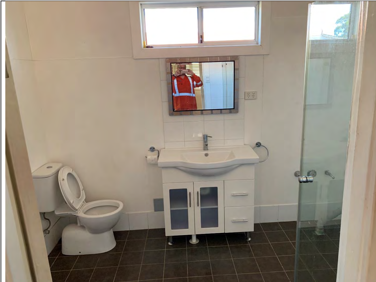
Photo 18 - View toward the south showing the bathroom (Room 3). The ceiling and the wall (partially covered by particle board) is composed of non-friable asbestos cement sheeting covered with lead-based paint.
