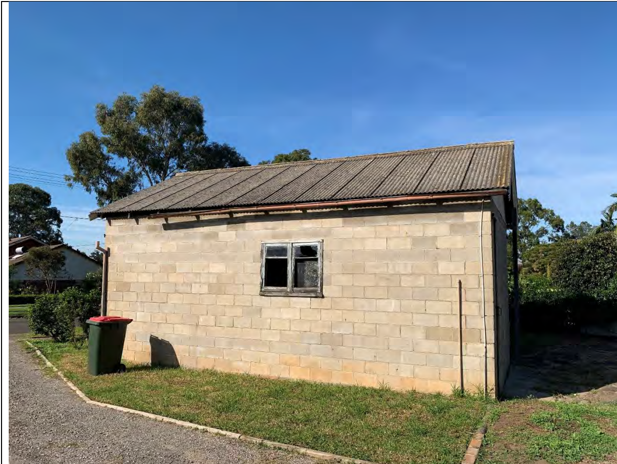
Photo 37 -View toward the south showing Garage #2. The roof is covered with non-friable asbestos cement corrugated roofing material. The gutter is presumed to be covered with red-coloured lead-based paint.
