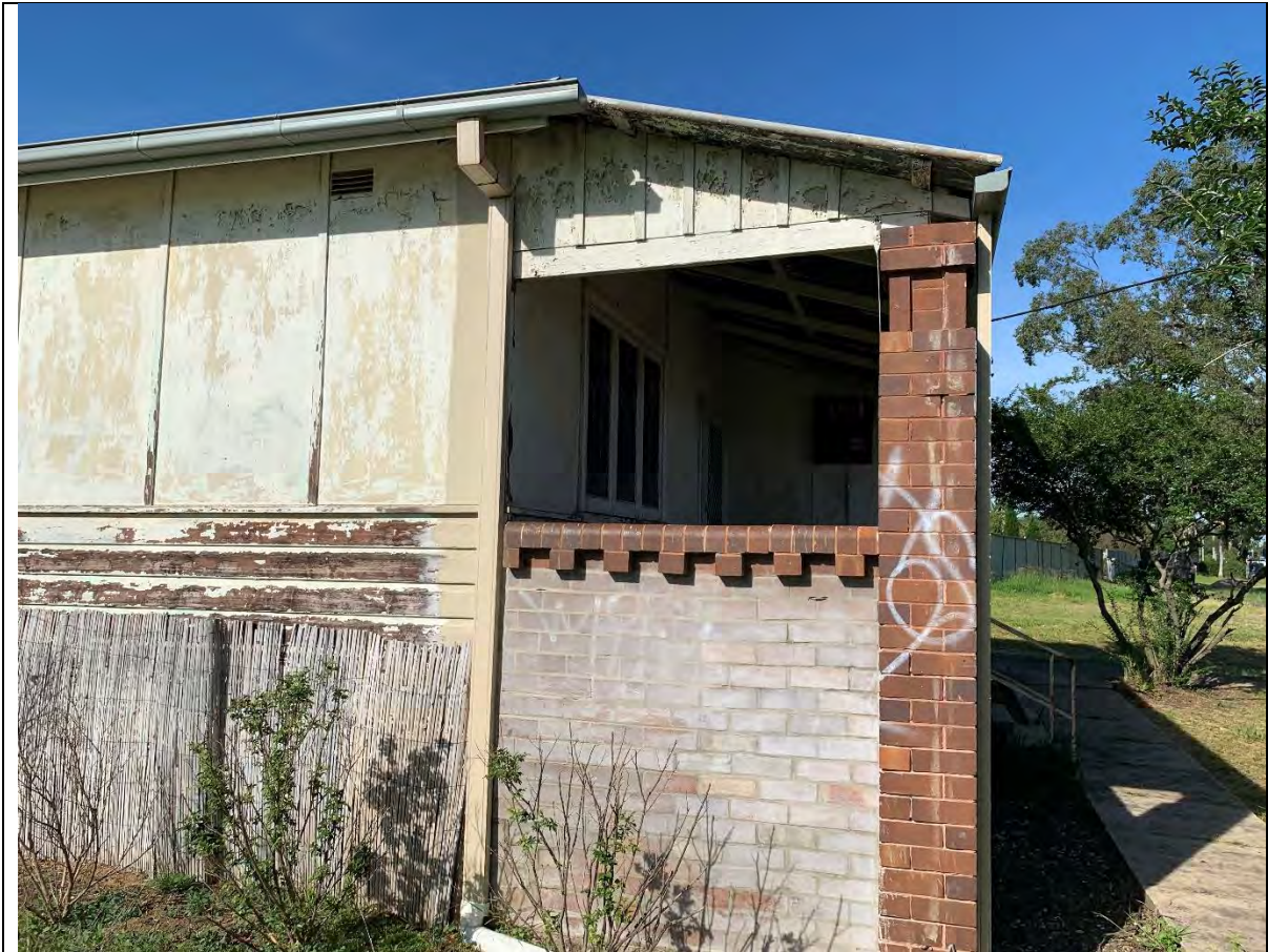
Photo 9 - View to the south showing the patio, the wood cladding covered with lead-based paint and the non-friable asbestos cement sheeting covered with lead-based paint.
