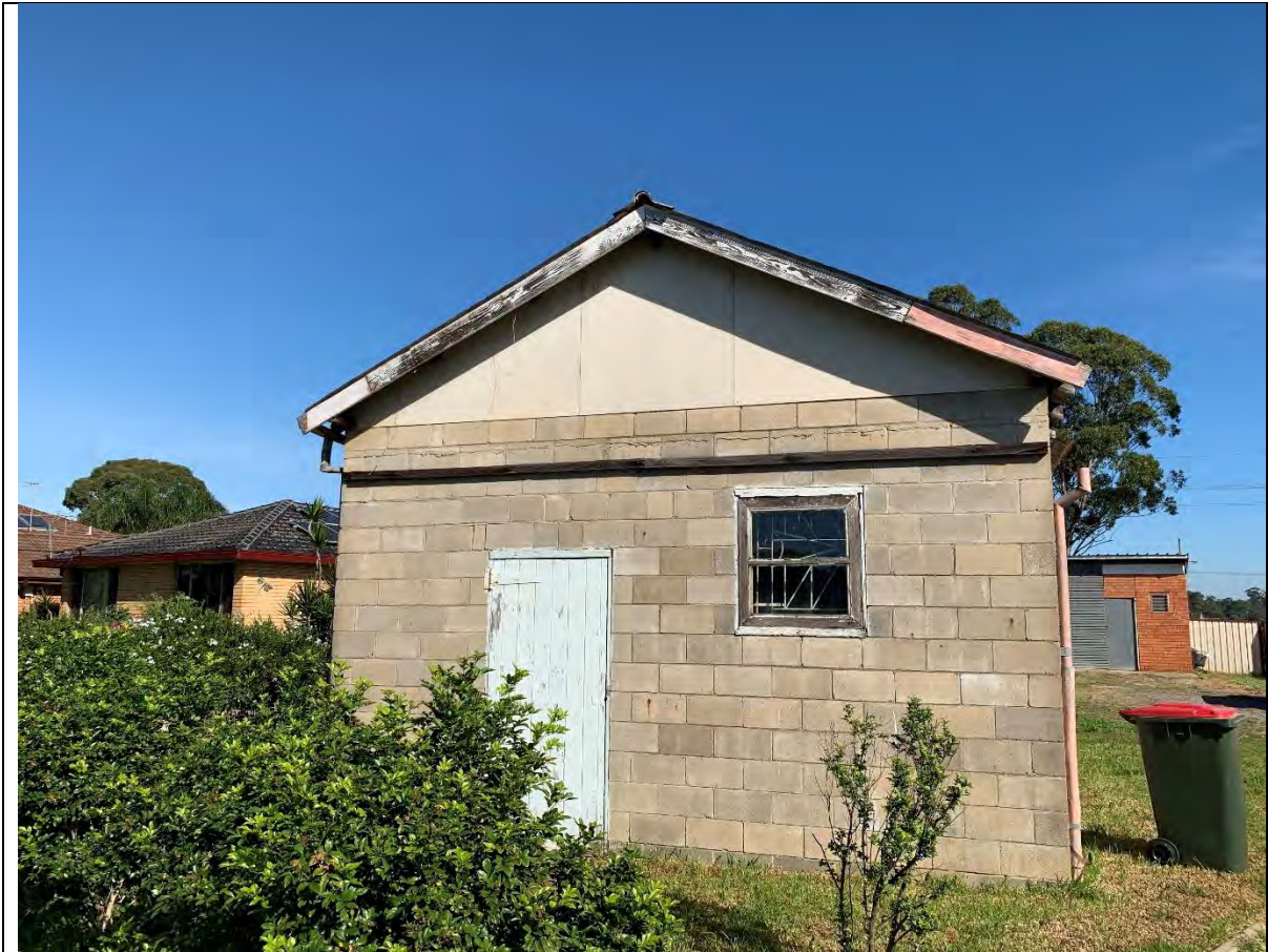
Photo 39 - View toward the west showing Garage #2. The roof is covered with non-friable asbestos cement corrugated roofing material. The gable is cladded with asbestos cement sheet cladding. The wood door and window frame are covered with lead-based paint.
