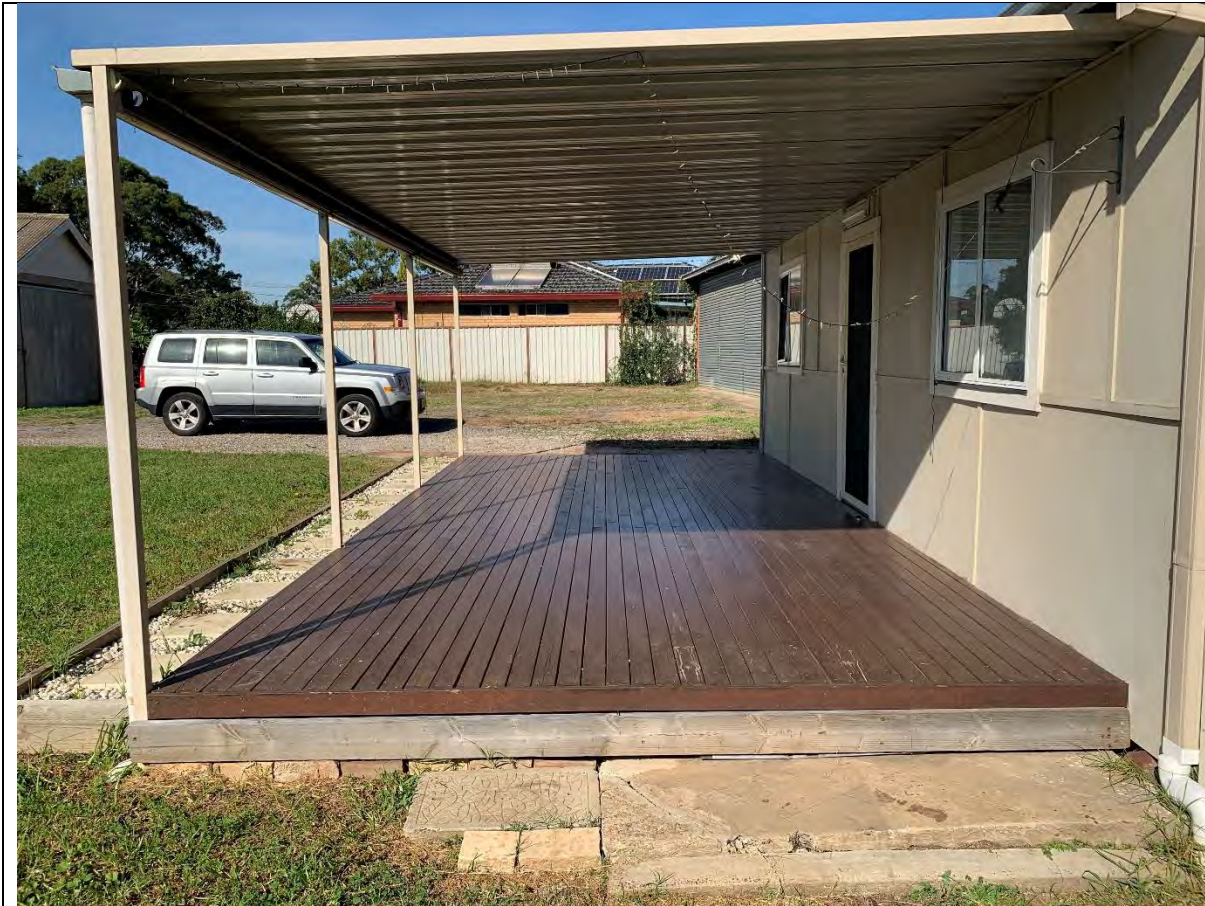
Photo 12 - View to the south showing the porch on the northern portion of the residence. The wall on the front of the house is covered with asbestos cement sheet cladding covered with lead-based paint.
