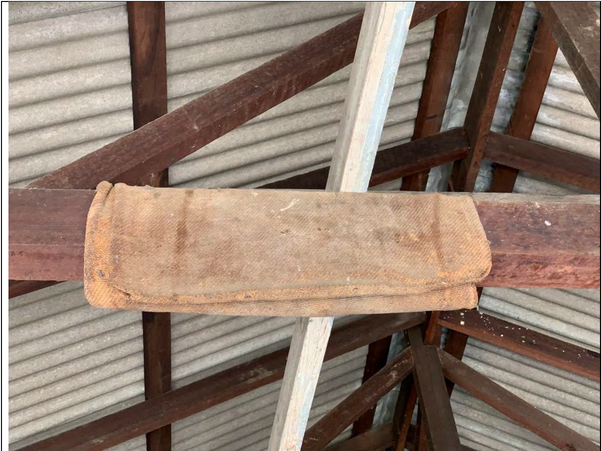
Photo 41 - View of the rafters and ceiling in Garage #2. A cloth presumed to be composed of asbestos material is present wrapped around the rafters. Corrugated asbestos cement roofing material is present on the ceiling.
