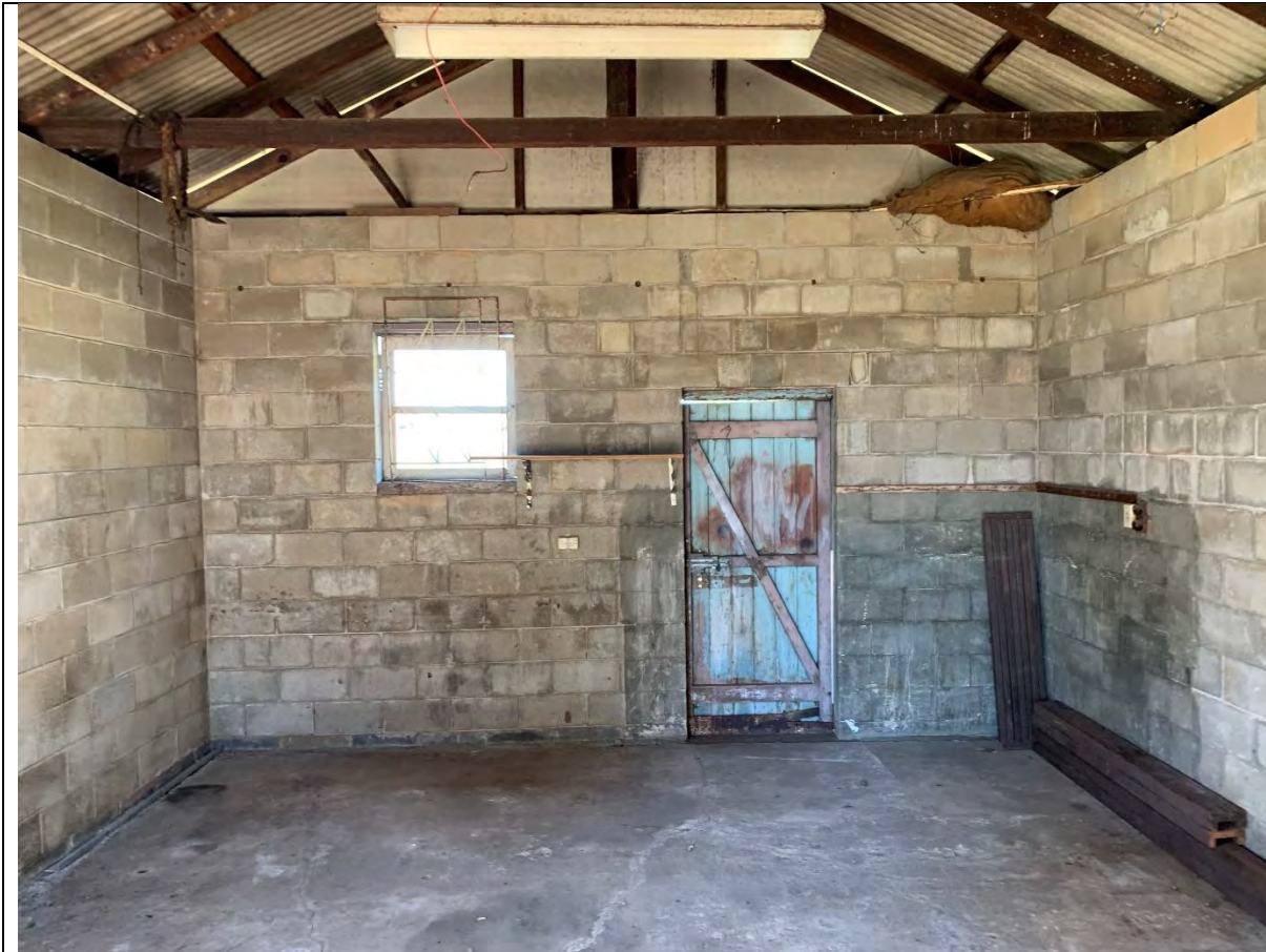
Photo 40 -View of the east side of the Garage # 2. A fluorescent light is shown on the ceiling. The wood door and window frame are covered with lead-based paint. A burlap bundle is present in the northeast corner in the rafters.
