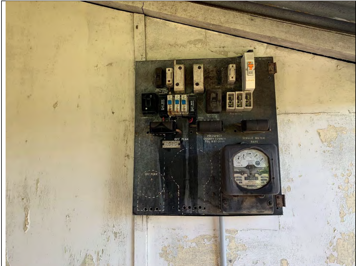
Photo 8 - View of electrical fuse box near porch on western side of the residence. Due to the age of the board ACM is presumed to be present
