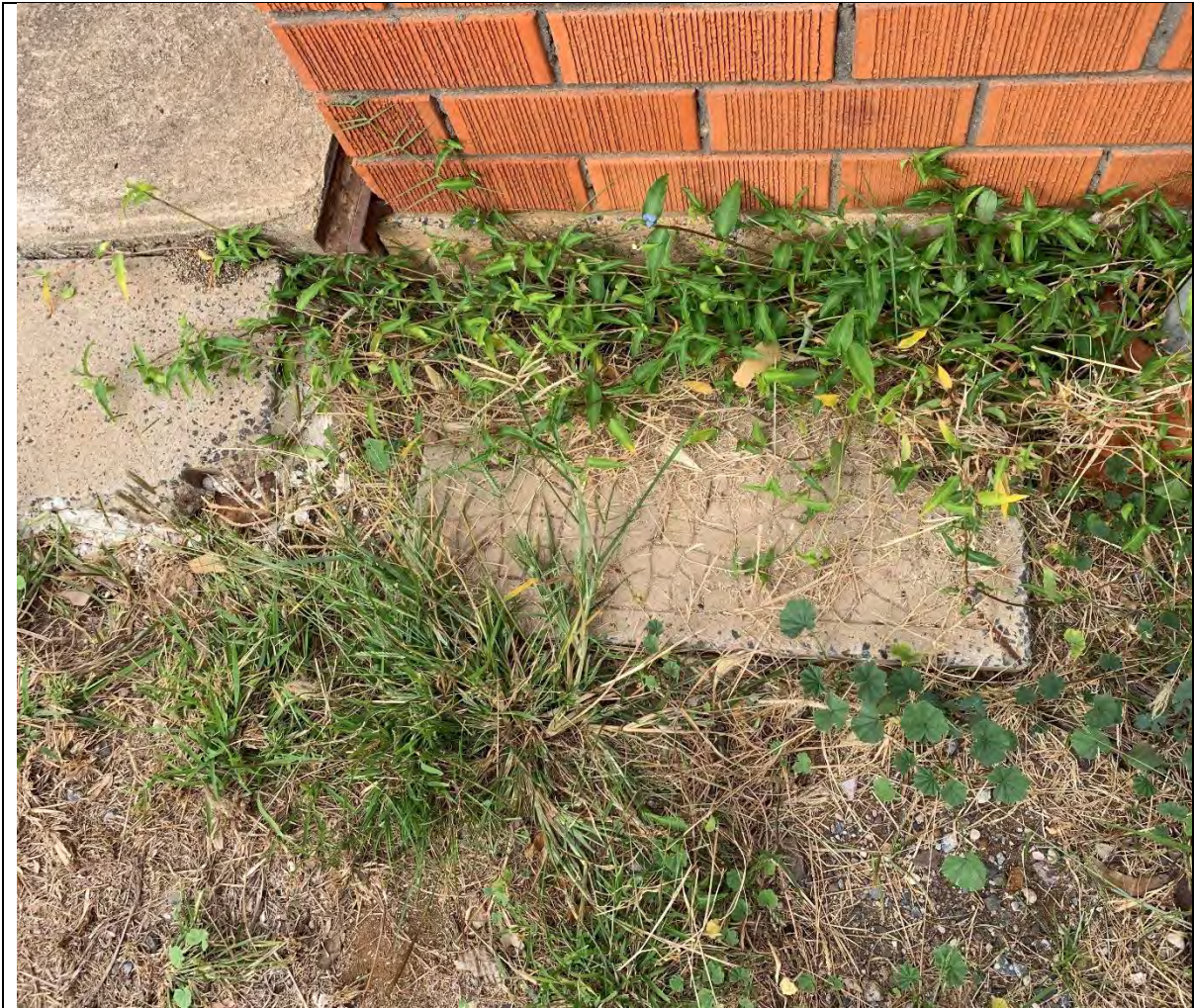
Photo 44 – View of the Telstra pit located adjacent to the wall on the north side of Garage #1. The pit may be composed of ACM.
