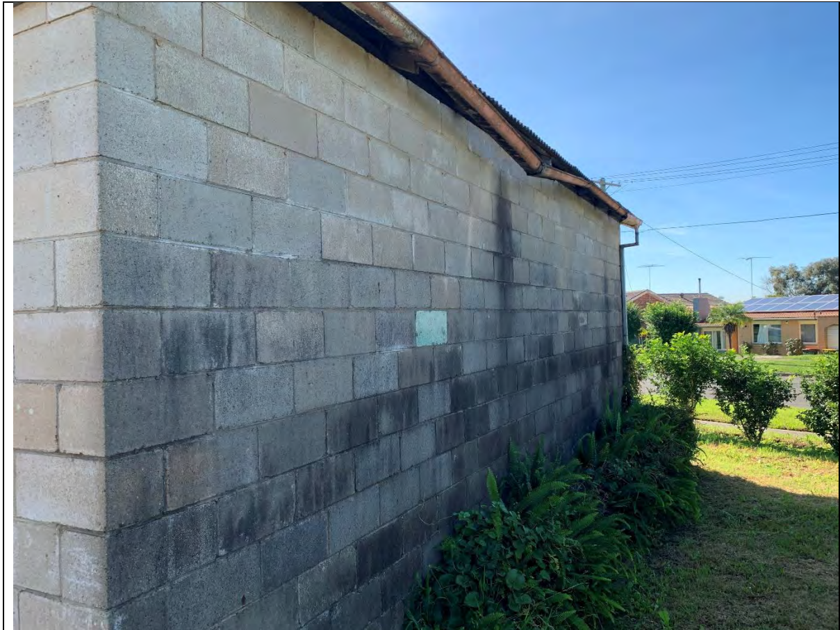
Photo 38 -View toward the east showing the east side of garage # 2. The gutter is presumed to be covered with red coloured lead-based paint.
