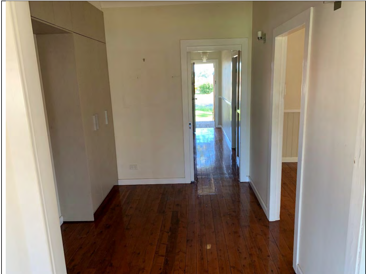
Photo 17 - View to the west showing the hallway. The walls and ceiling are covered with lead-based paint. The floor is composed of wood. The walls and ceiling are composed of gyprock.
