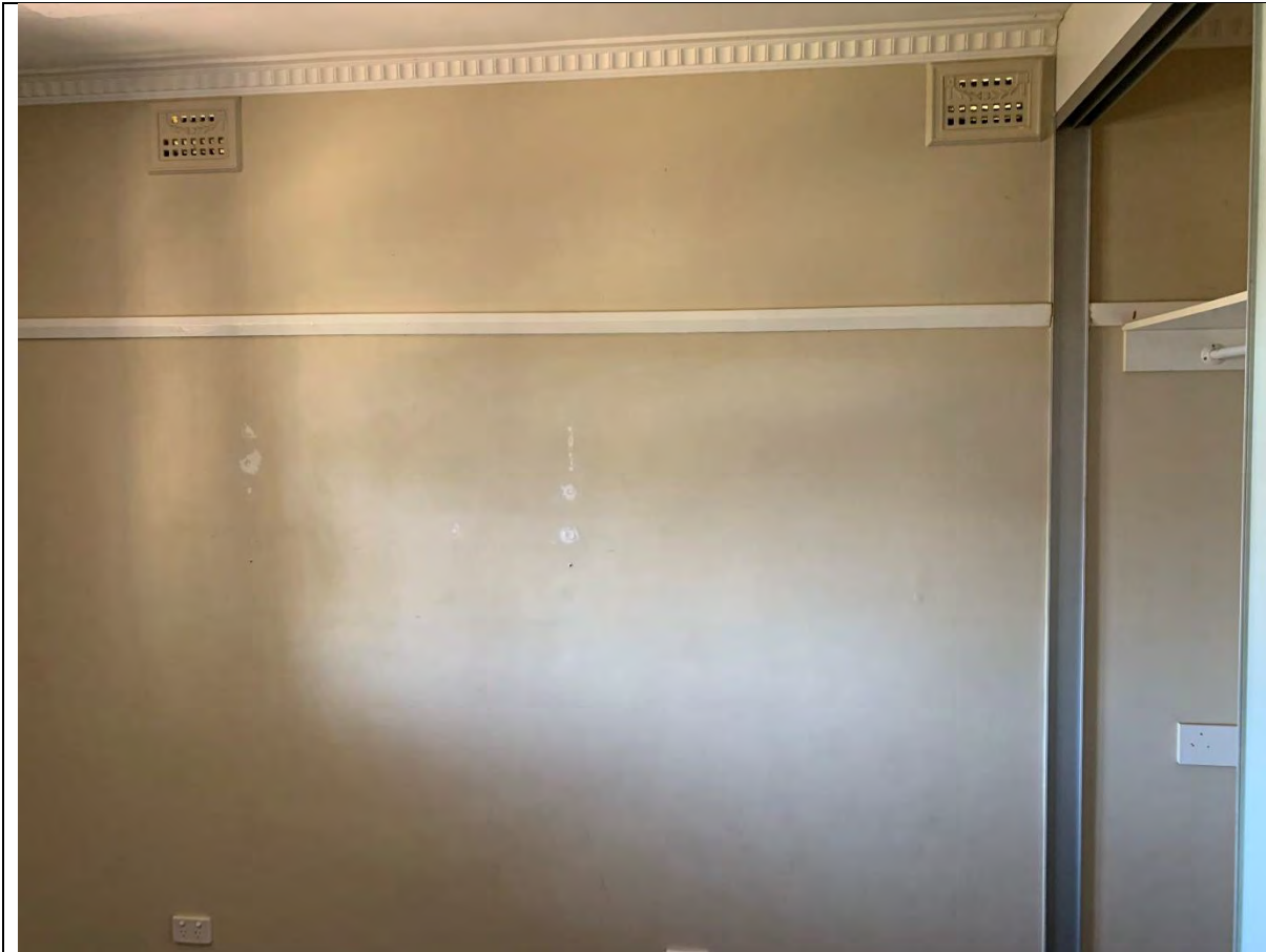
Photo 22- View towards the west showing the wall and closet in Room 5. The walls and ceiling are composed of gyprock and are covered with lead-based paint. The floor is composed of wood.
