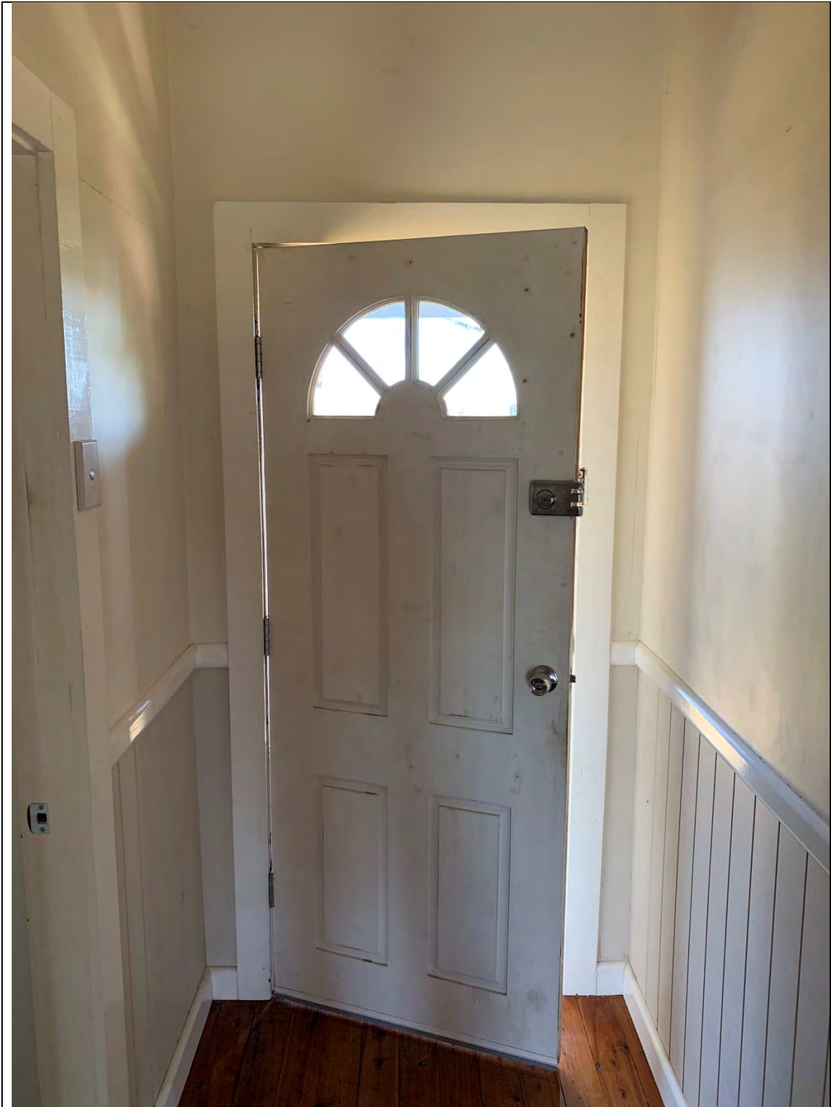
Photo 27 - View towards the west showing the door located on the southern side of the site. The door, walls and ceiling are covered with lead-based paint.
