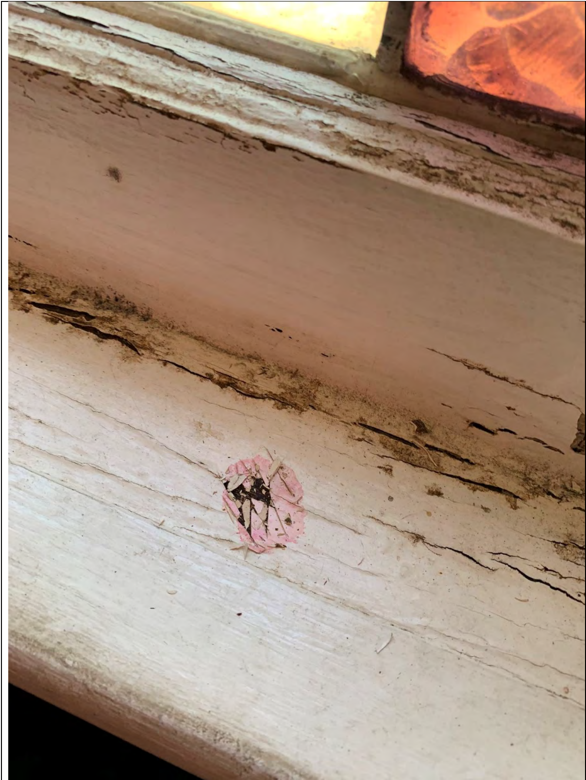
Photo 26 - View of the window frame surrounding the stained-glass window in Room 7. The wood window frame is covered with white lead-based paint.
