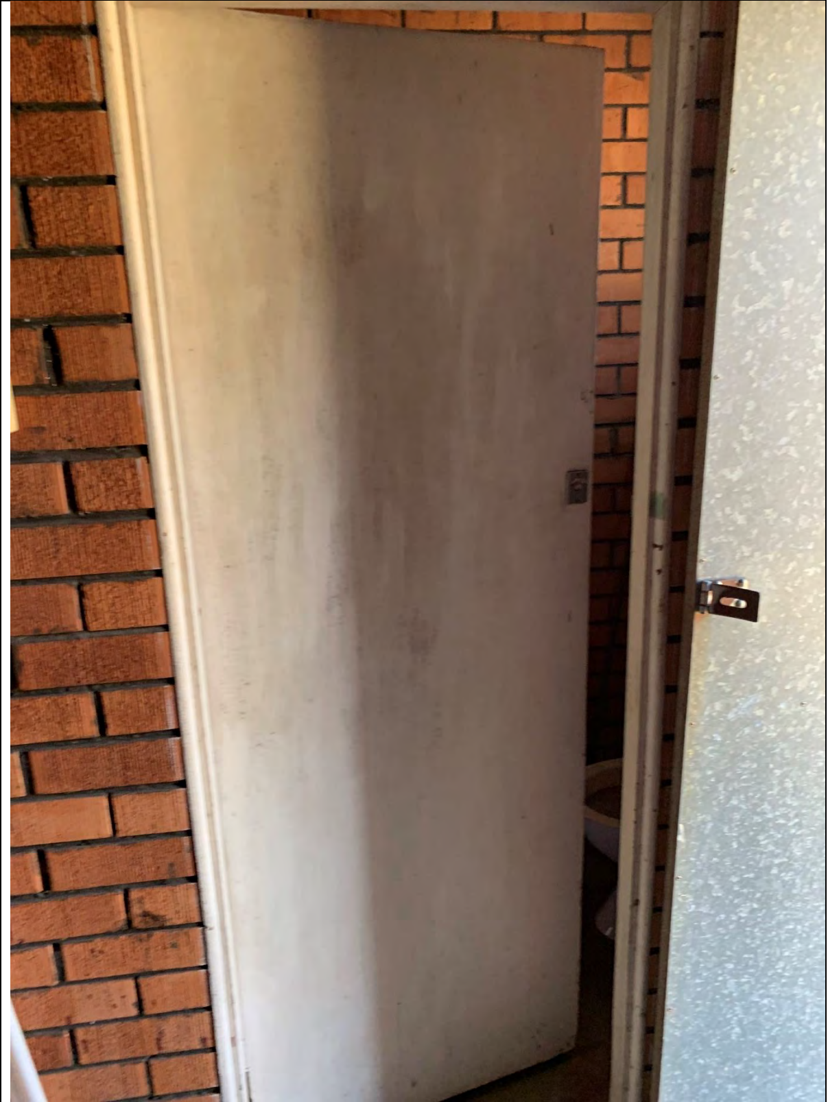
Photo 35 - View of the bathroom door in Garage # 1. The door is covered with lead-based paint.
