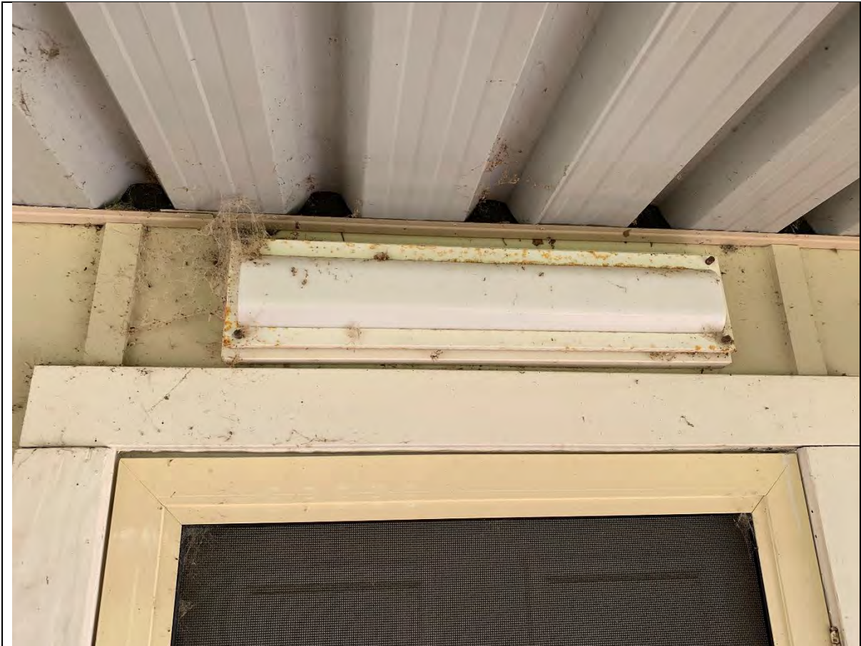
Photo 14 - View of a fluorescent light located above the door on the eastern side of the residence. The wood trim is presumed to be covered with lead-based paint.
