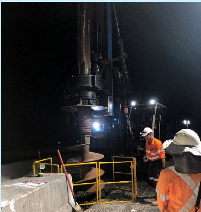
Right: Piling rig in place for the pillar of the new bridge over the M4 completed in March.
