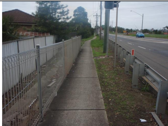
Photo A4, concrete footpath eastern side of Prospect Highway, south of Harrod Street, towards south
