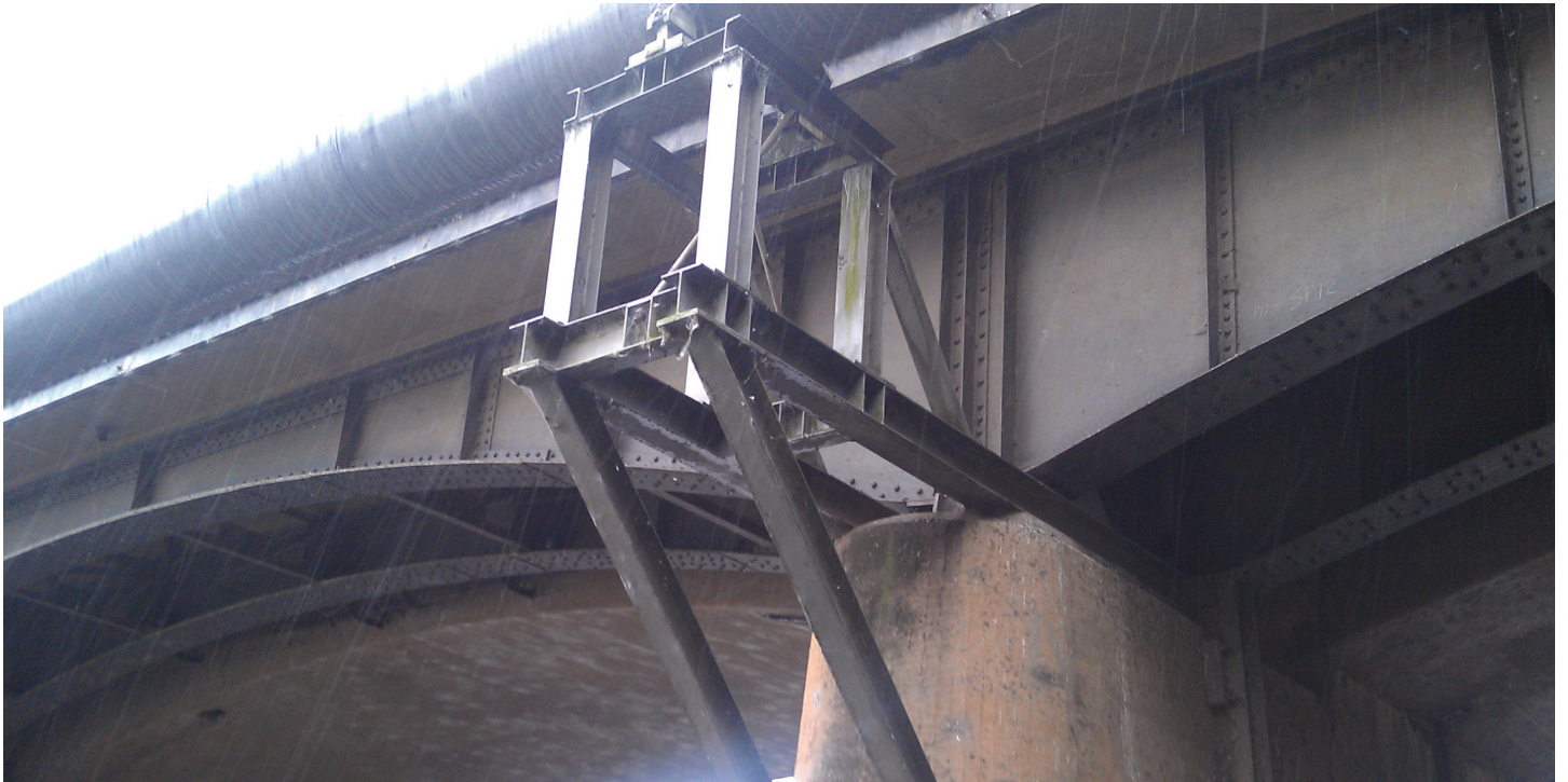
Support structure of the water main on the downstream side of Richmond Bridge
