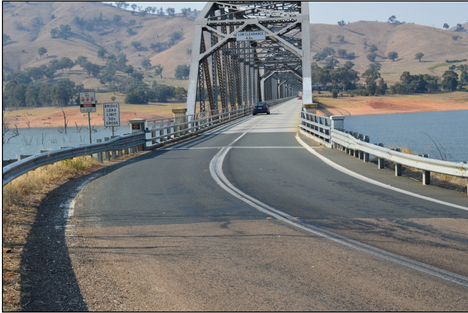
Plate 2: The NSW Approach to the Bethanga Bridge looking southeast and showing modification made in 2005. Note repainting on steel trusses to cover graffiti.
