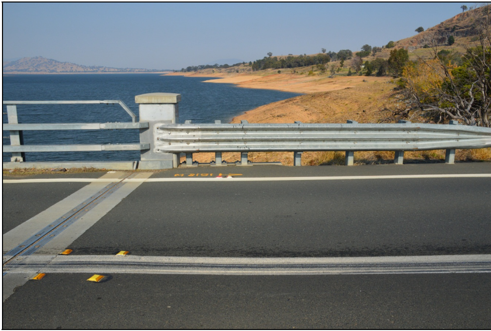
Plate 3: Detail of the NSW road approach and west end of the Bethanga Bridge looking southeast showing abutment to which the bridge guard rails and road barriers is attached, also note spray painted construction markings on road possibly signifying limit of works of proposal.
