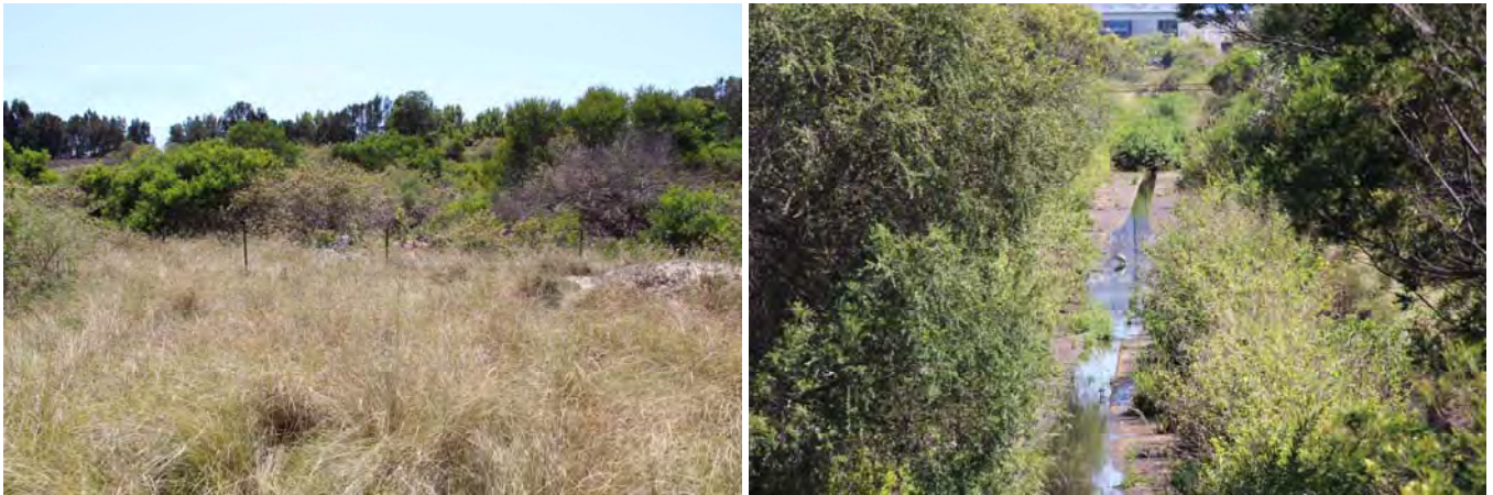
View east to railway embankment (L) and concrete lined drainage channel (R)
