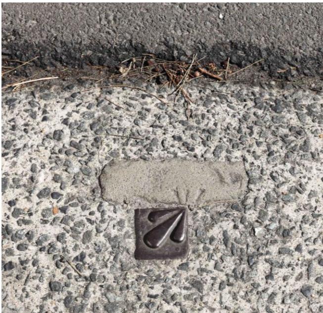
Image 5.21. Detail of the alignment pins at McBurney Avenue and Botany Road. Facing west. Stedinger Associates 2014. Image 2159.
