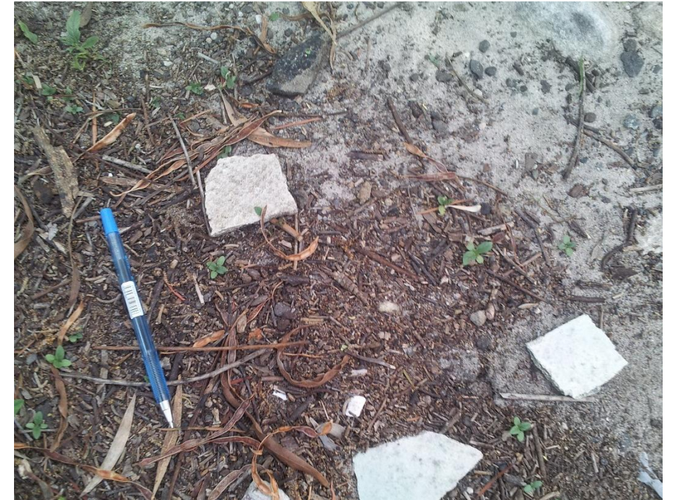
Photograph 3 – Asbestos fragments along southern boundary.
