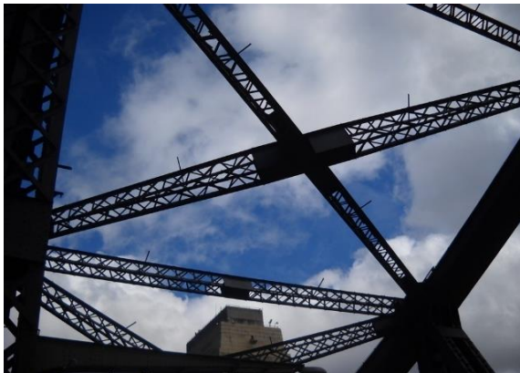
Figure 22: View up from bridge deck showing the distinctive significant pattern formed by the arch trusses. (Source: Roads and Maritime)
