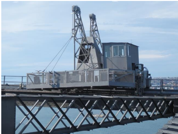
Figure 16: View east along top of the arch towards an existing AMU operating on the east top chord. (Source: Roads and Maritime)
