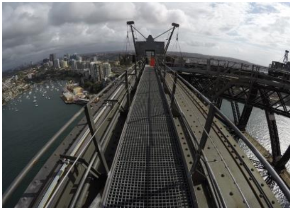
Figure 23: View across existing SHB walkway showing fibreglass mesh (Source: Roads and Maritime)
