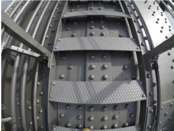
Figure 24: Detail shot of original steel stair treads on existing SHB walkway. (Source: Roads and Maritime)
