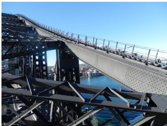
Figure 12: View north east along the top of the arch towards the east top chord stairway. (Source: Roads and Maritime)
