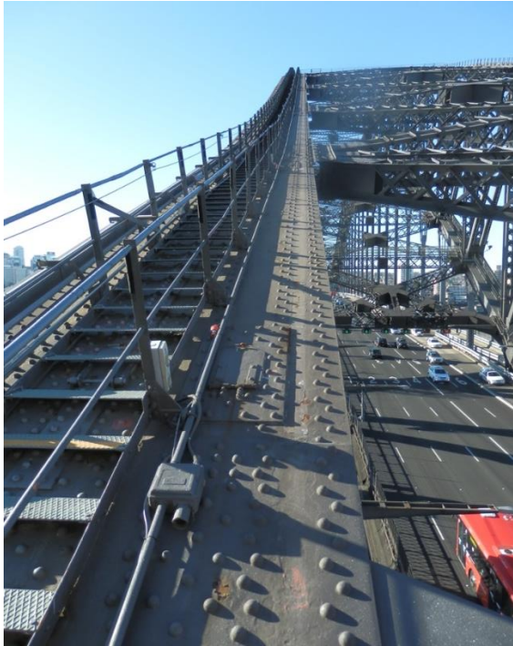
Figure 14: View north east along the west top chord of the arch showing metal stairs. (Source: Roads and Maritime)
