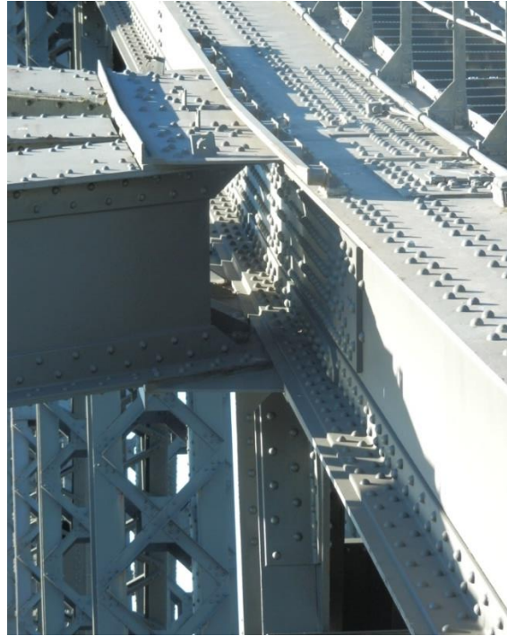
Figure 15: Detail shot of rivets on the east top chord near the metal stairway. (Source: Roads and Maritime)
