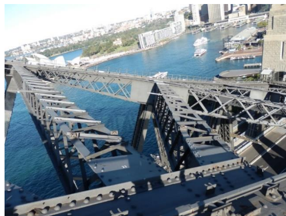
Figure 13: View south east along lateral truss members from west top chord stairway. (Source: Roads and Maritime)
