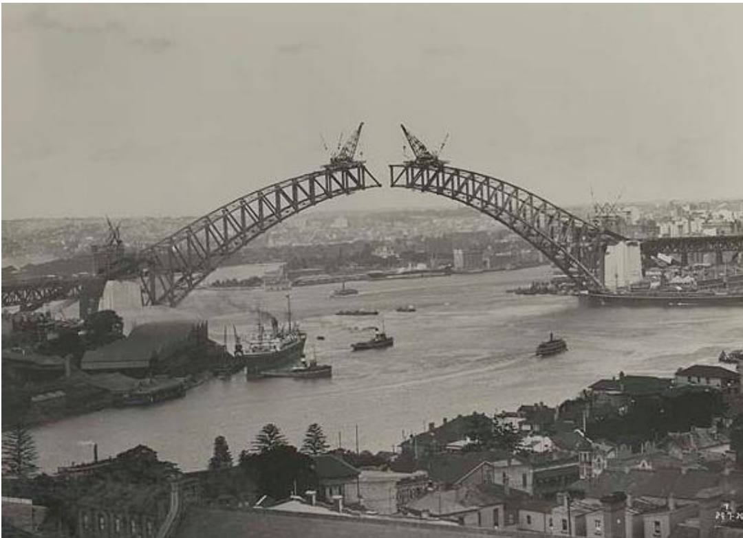
Figure 7: Construction of SHB showing creeper cranes in place, 1930. (Source: State Records NSW, Digital ID: 12685_a007_a00704_8729000194r)
