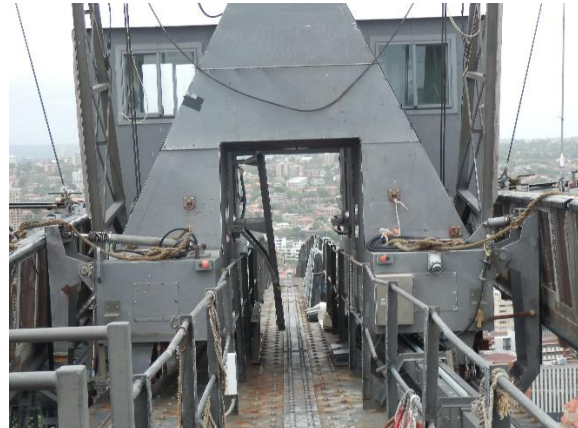
Figure 17: View north east towards existing AMU operating on the east top chord overhead walkway. (Source: Roads and Maritime)
