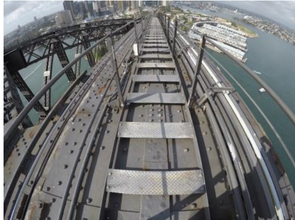
Figure 25: View down existing SHB walkway showing modern checker plate stair treads. (Source: Roads and Maritime)
