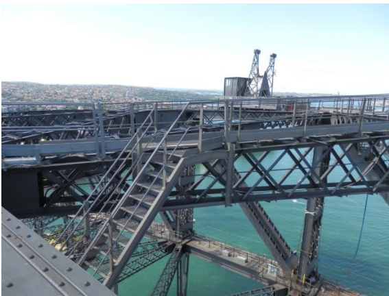
Figure 20: View northeast across trusses towards an existing AMU operating on the east top chord. Catwalks seen in foreground. (Source: Roads and Maritime)
