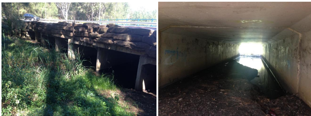
Figure 3-2 The box culverts under the Glenmore Parkway showing entrance and internal view (camera flash not used to show light conditions inside culvert)
