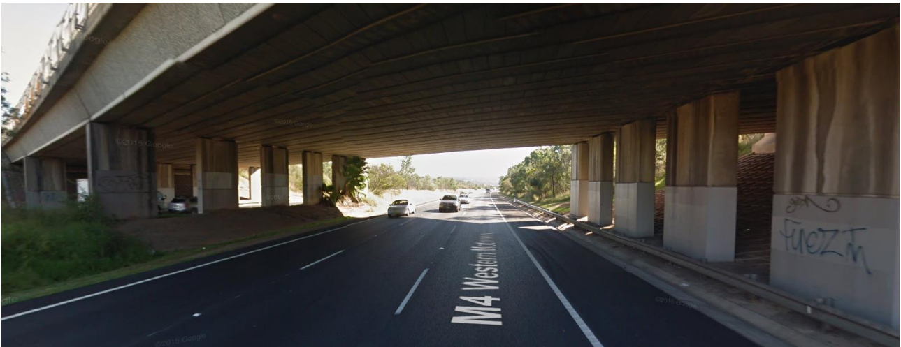
Figure 3-3 The Northern Road bridge over the M4 Motorway (source: Google street view)
