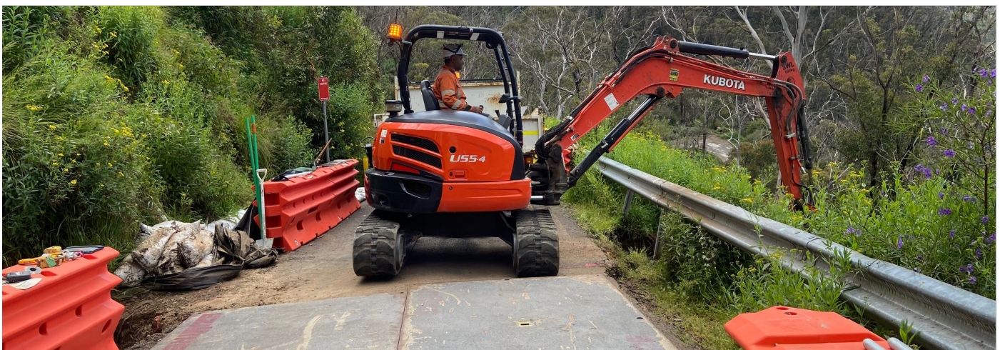
Installing a new culvert on the Two Mile section of Jenolan Caves Road in November
