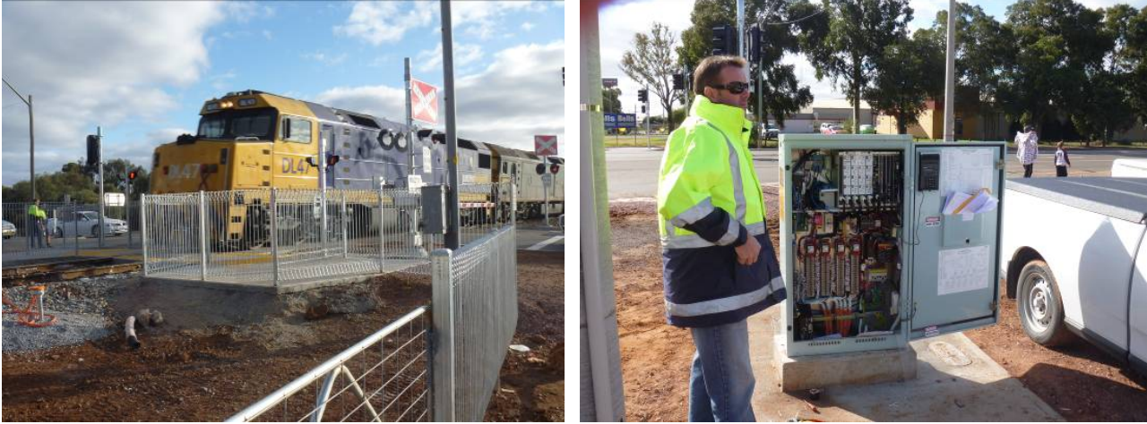
Figure 4: Construction of level crossing and traffic signal interface at Canal Street, Leeton.
