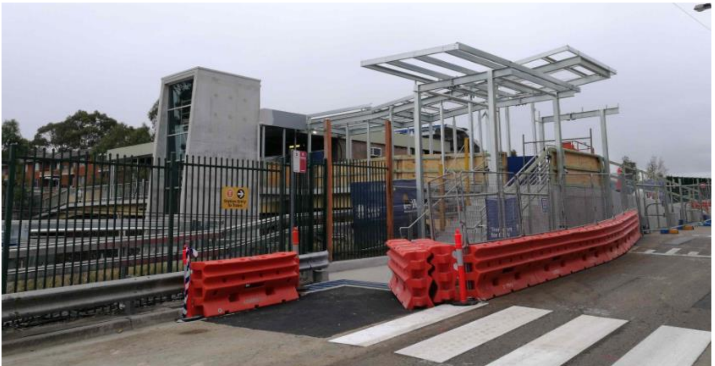
November 2017- Lift shaft erected, new station entry stairs, ramp and relocated crossing on Station Street West.
