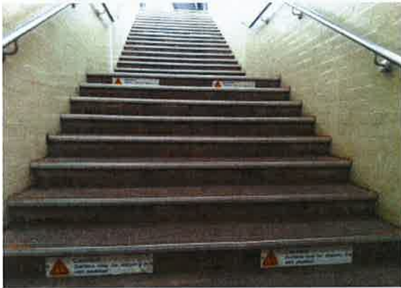
Only stair access to the station is currently provided
