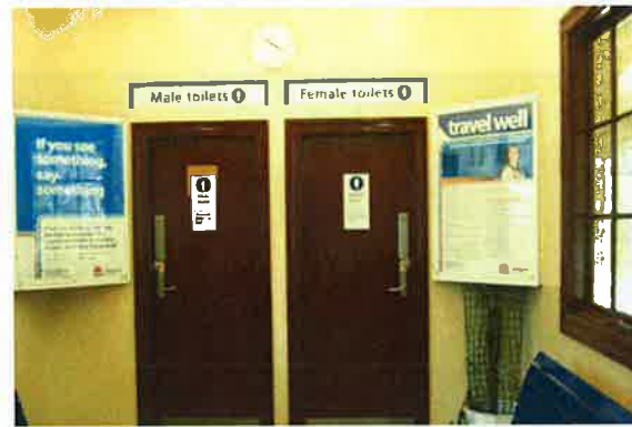
Toilets off the Waiting Room are not DDA compliant
