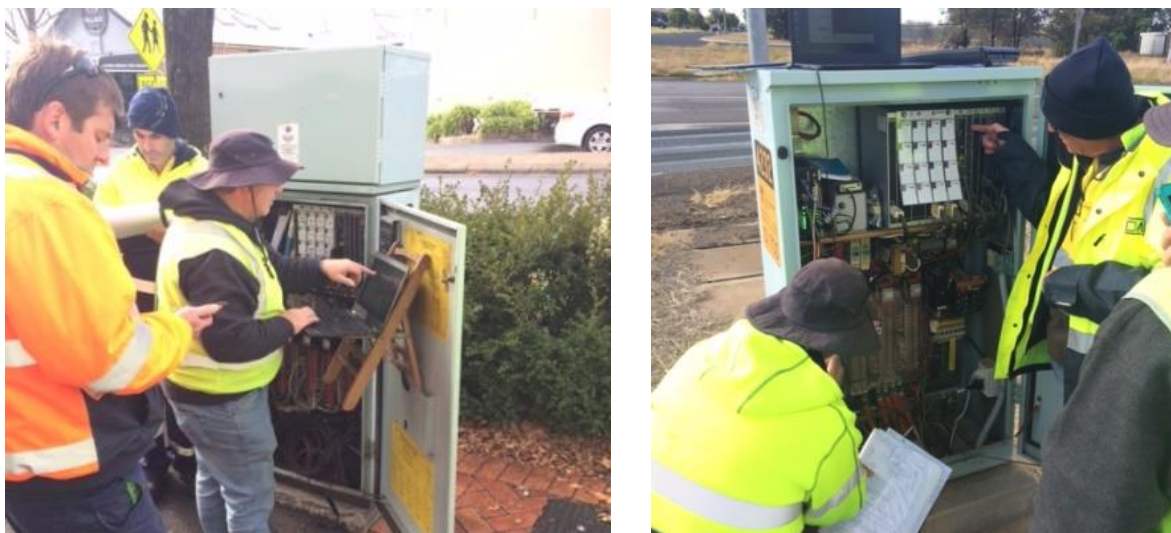
Figure 1: Roads and Maritime and RIMs joint testing of the interconnected level crossings at Orange (L) and Parkes (R)
