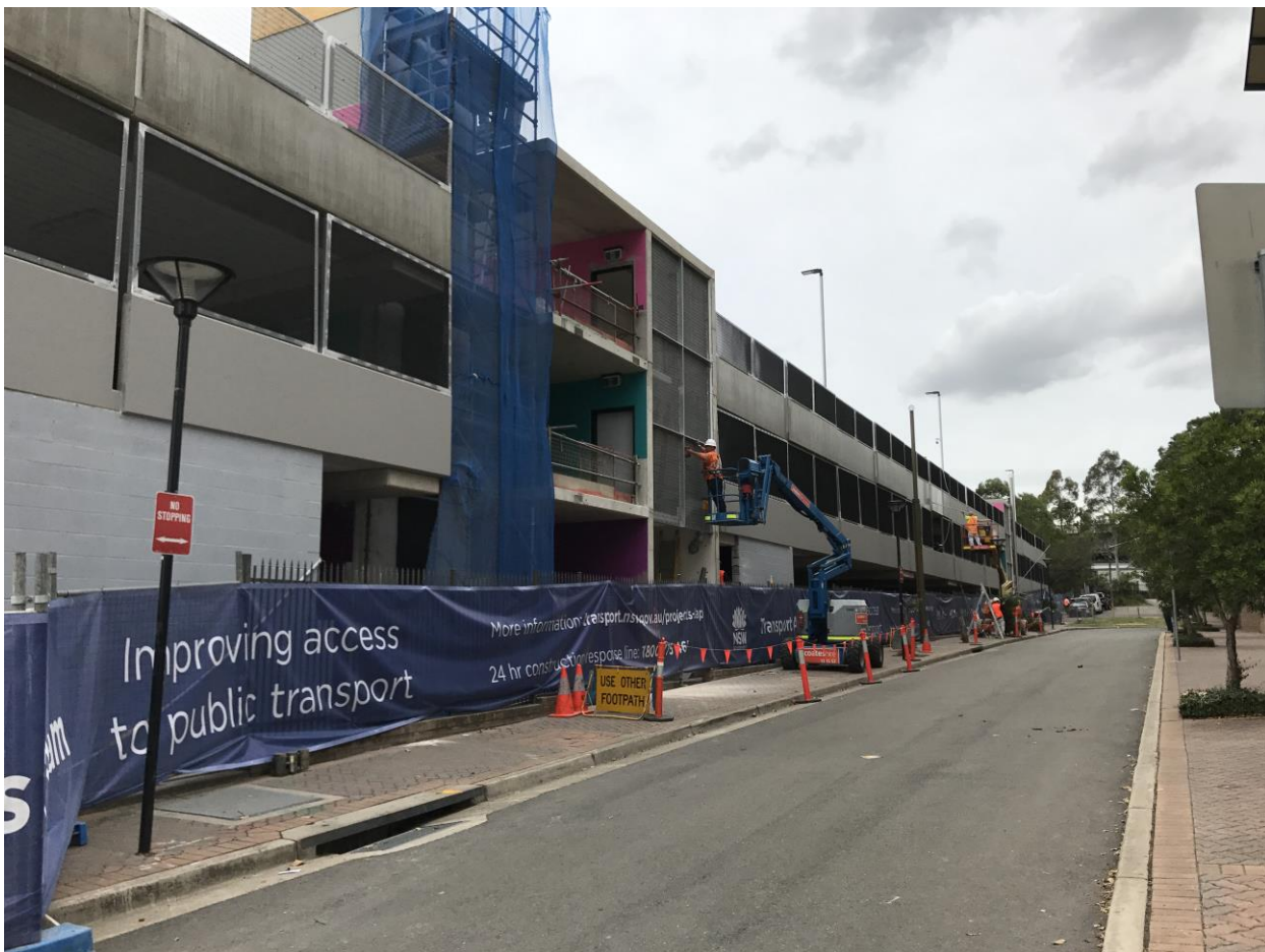
View of construction of Ashfield Commuter Car Park from Brown Street – February 2018
