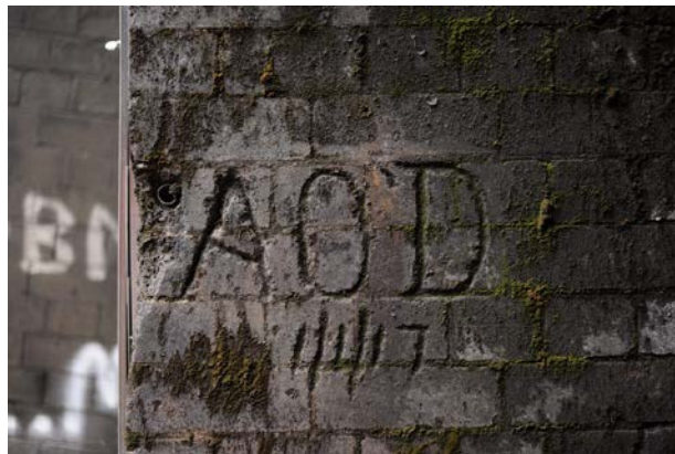
Figure 117: Detail shot of Tunnel 10 Lithgow end up track portal entrance showing engraving in brickwork
