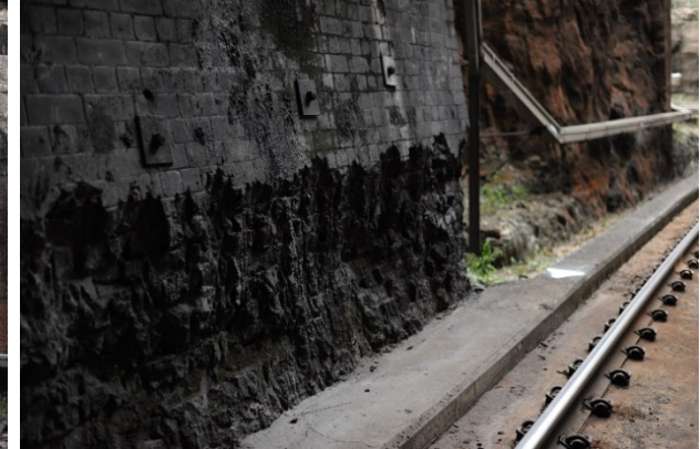
Figure 80: Detail of existing toe notching and rock bolts, down track, Lithgow end portal
