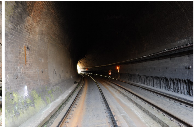
Figure 45: Internal view of Tunnel 2 showing existing toe notching on down track
