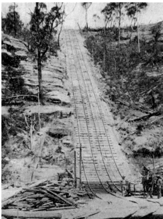
Figure 7: Funicular used to carry materials in the construction of the Great Zig Zag Railway deviation tunnels to the Lithgow end of Tunnel 9 (Source: NSW Railway and Tramway Magazine)
