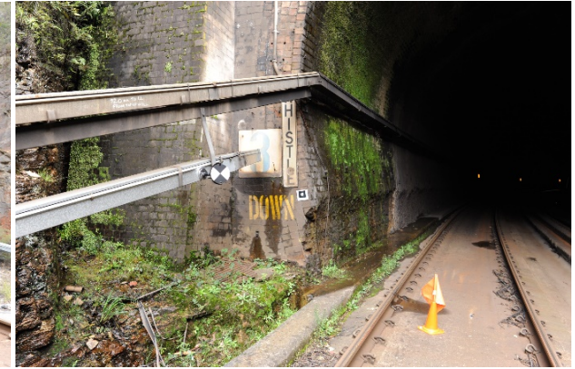
Figure 54: Detail photo of GST and existing notching, down track Sydney end portal
