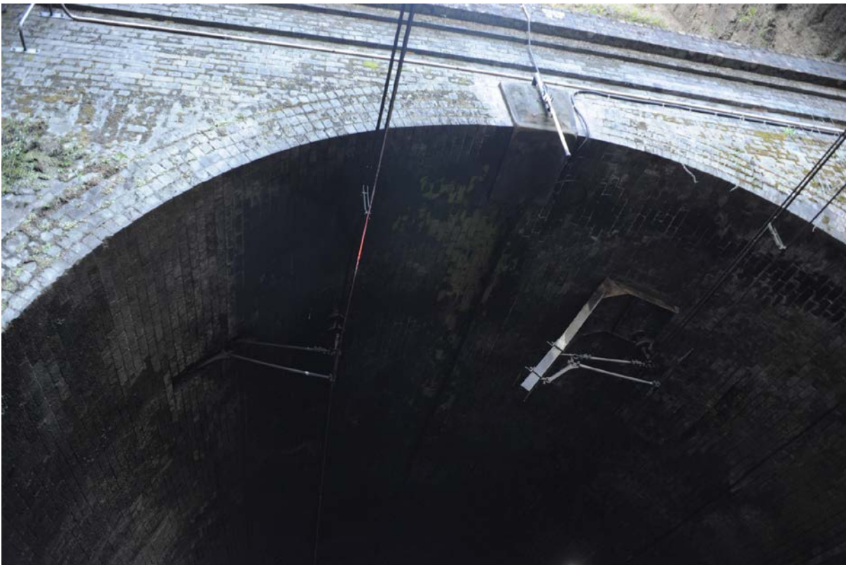
Figure 19: Overhead wiring structures on the brick vault of Tunnel 1, Lithgow end portal
