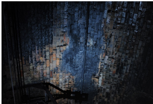
Figure 38: Detail of water seepage through brick vault
