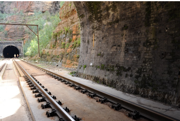
Figure 72: View from Lithgow end portal looking towards Sydney end portal of Tunnel 6
