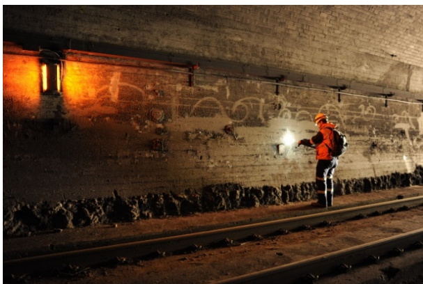
Figure 89: Internal view of Tunnel 7 showing existing toe notching and lighting, down track
