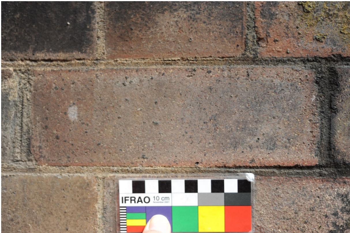
Figure 15: Example of English Cross bond from the country end portal of Tunnel 8
