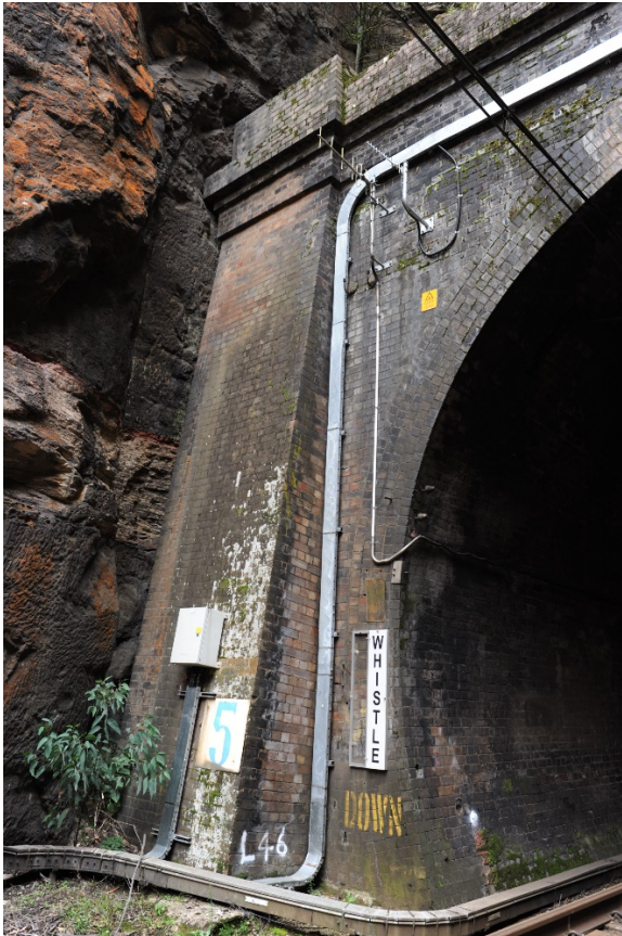
Figure 75: Detail shot showing communication cabling and GST on Sydney end portal, down track
