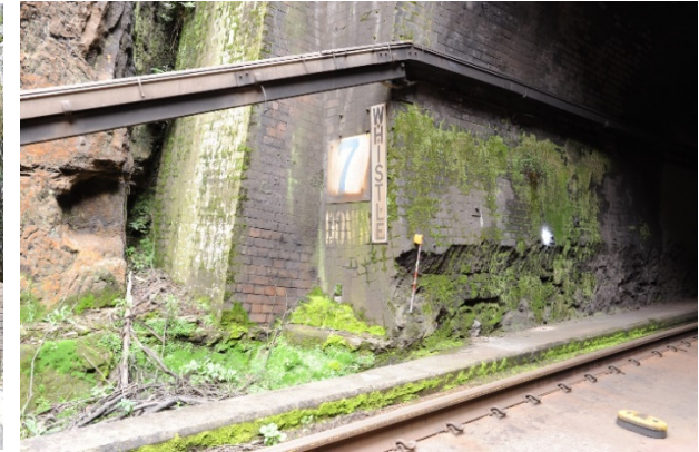
Figure 88: Detail photo of GST and existing notching, down track Sydney end portal
