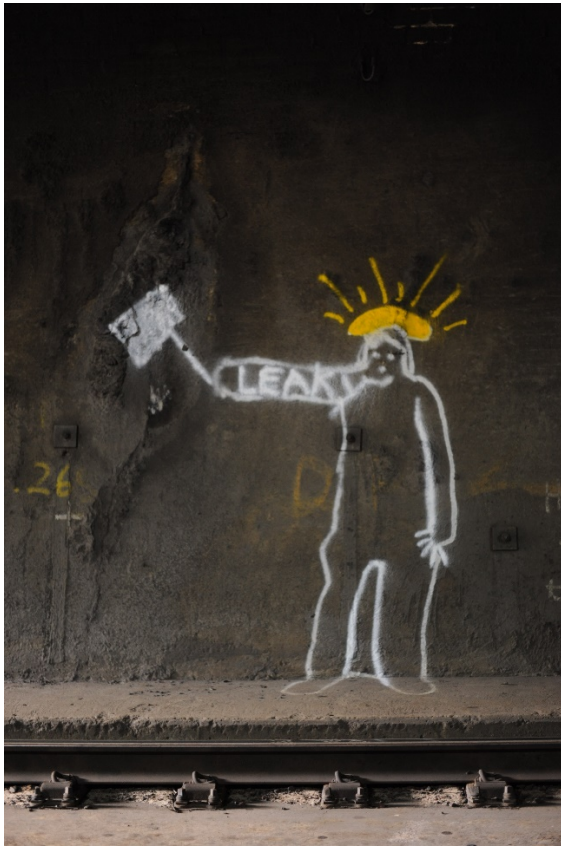
Figure 119: Detail shot showing graffiti and existing rock bolts within Tunnel 10
