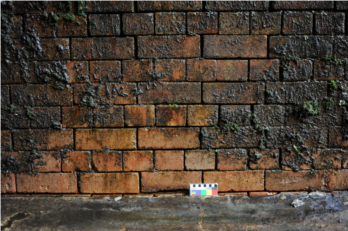
Figure 16: Example of English Cross bond from the city end portal of Tunnel 1, showing where water has removed some of the concrete bonding
