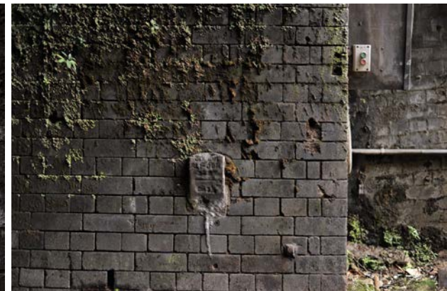
Figure 118: Detail shot of Tunnel 10 Lithgow end down track portal entrance showing gradient/radius/survey marker
