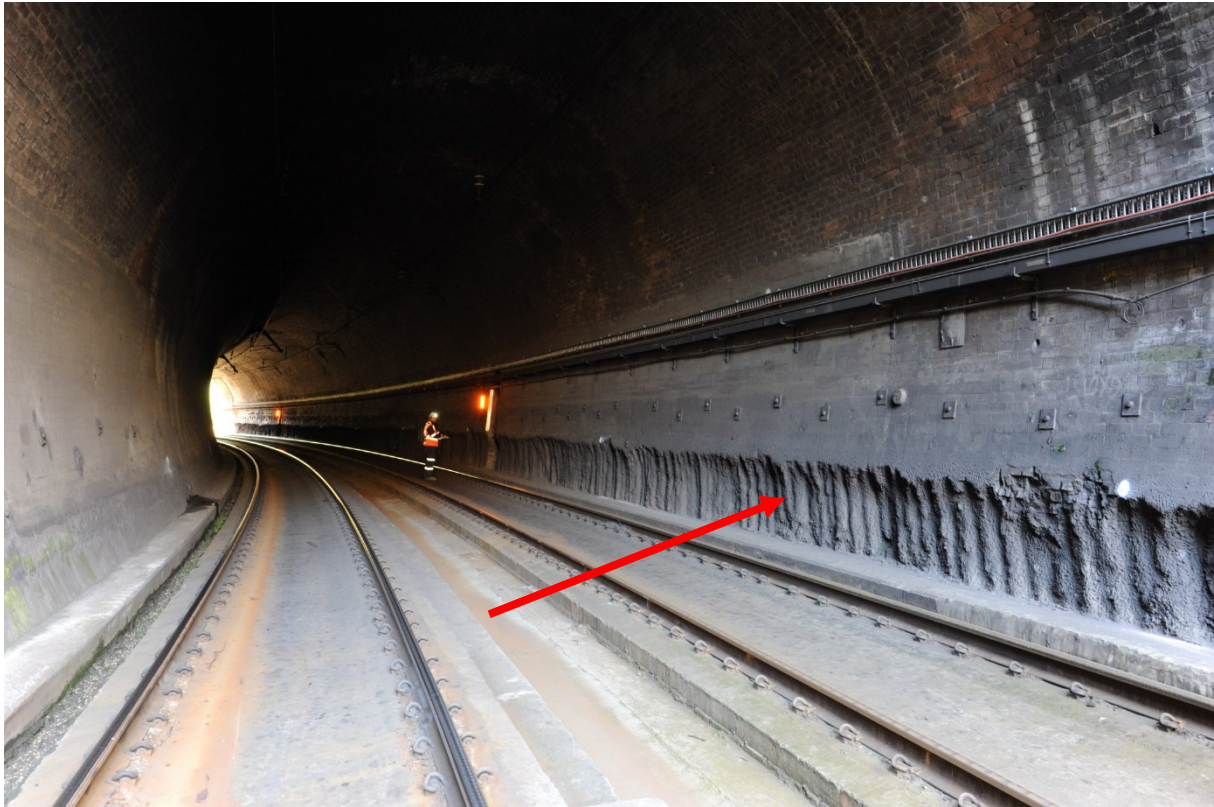
Figure 14: View up track within Tunnel 9, showing concrete track bed and notching at the toe of the tunnel wall from track bed lowering in the 1970s. Tunnel 9 is the only tunnel that is wholly lined with bricks (red arrow indicates previous notching).
