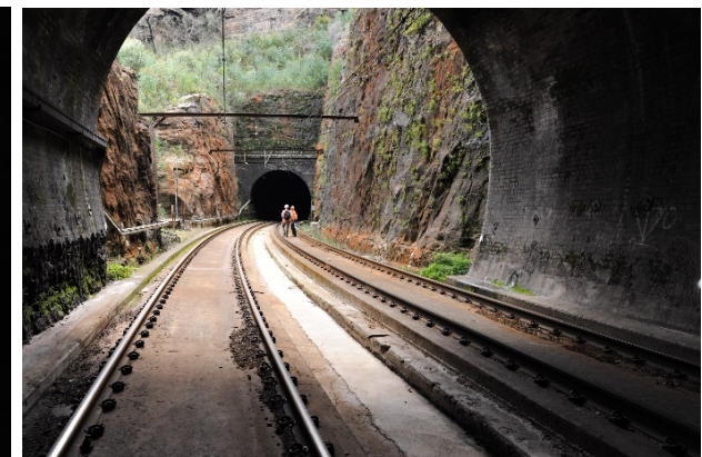
Figure 83: View from Lithgow end portal of Tunnel 6 towards Sydney end portal of Tunnel 7
