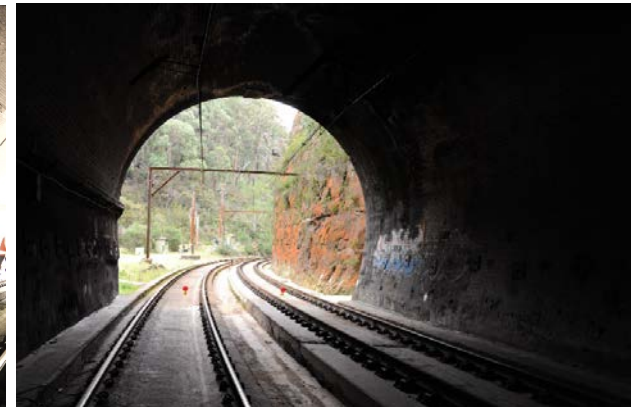
Figure 109: View out from Tunnel 9 towards country end portal and compound area beyond
