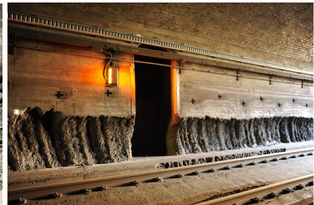
Figure 48: Existing toe notching on down track showing internal 'recess' in tunnel wall
