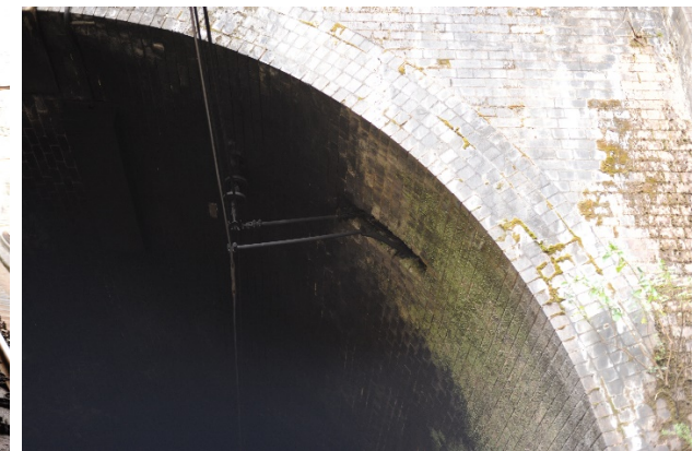
Figure 100: Detail of overhead wiring structures at Tunnel 8
