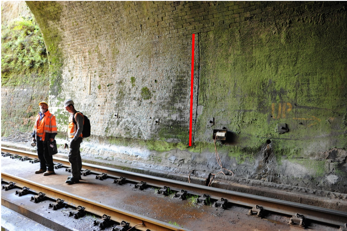
Figure 13: Country end of Tunnel 1, showing brick tunnel portal and transition to concrete across the lower tunnel wall approximately six metres from the portal (red line placed adjacent to change from brick to concrete to highlight the interface)
