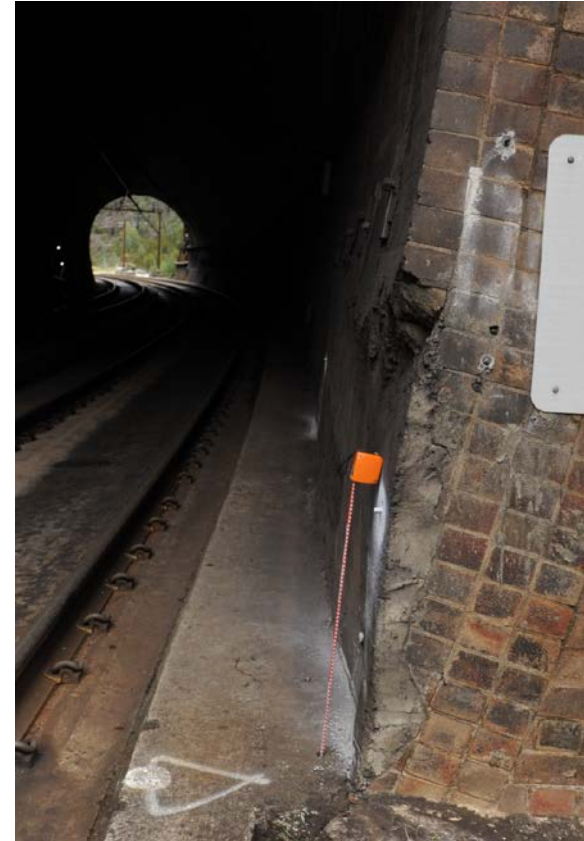
Figure 112: Lithgow end portal, down track, showing removal of up to three courses of brick during previous notching of tunnel lining
