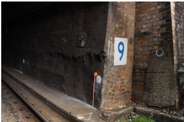
Figure 107: Detail shot of existing toe notching and rock bolts, Lithgow end portal, down track
