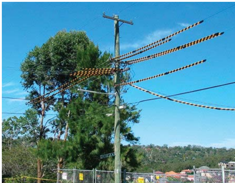
Figure 127: Example of Tiger Tail protection installed on a transmission line
