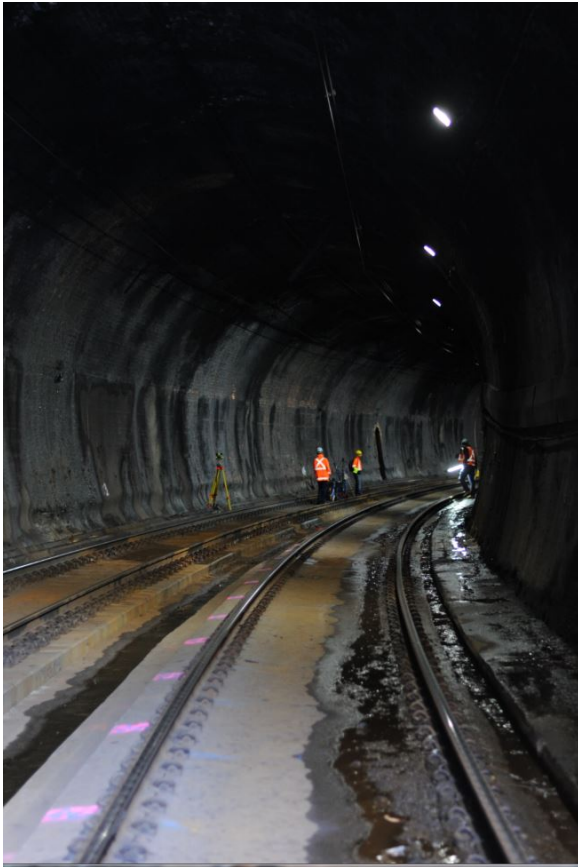
Figure 40: Tunnel 1, showing existing toe notching on the up track tunnel lining
