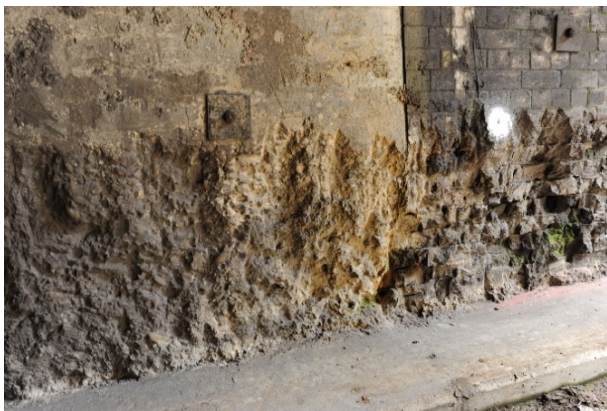
Figure 81: Detail of existing toe notching and rock bolts, showing original concrete (left) and brick (right) fabric
