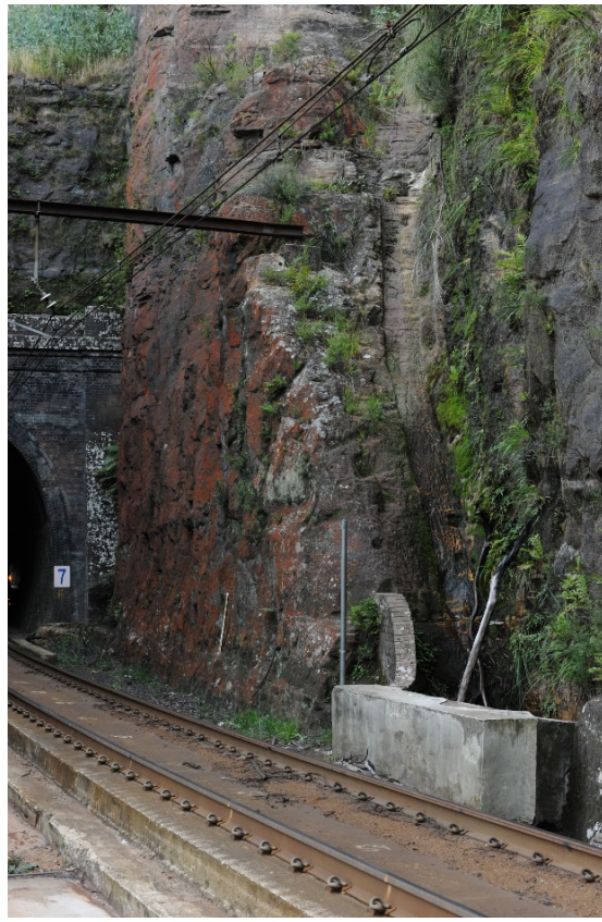
Figure 93: Detail shot of original drainage features near Sydney end portal of Tunnel 7
