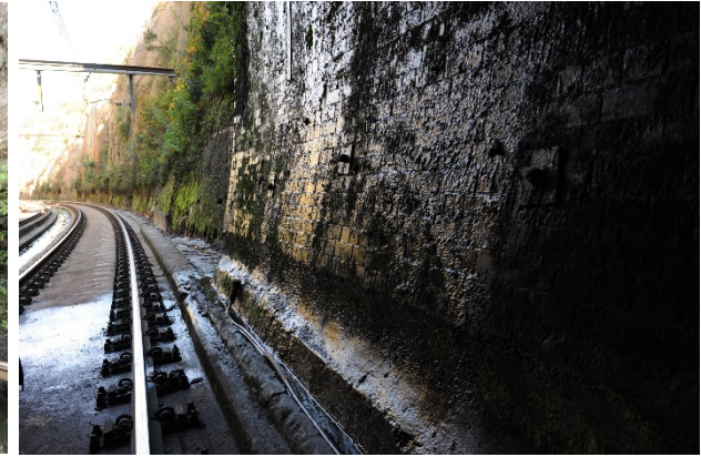
Figure 36: Detail of existing notching, up track Lithgow End
