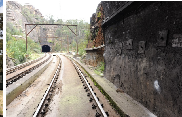
Figure 106: Detail of rock bolts and toe notching, Sydney end portal, down track
