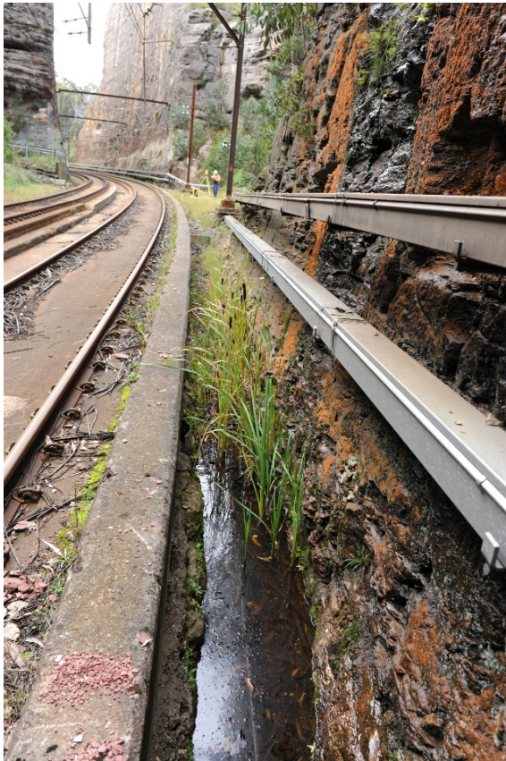
Figure 58: GST attached to sandstone cutting, down track, adjacent to Sydney end portal
