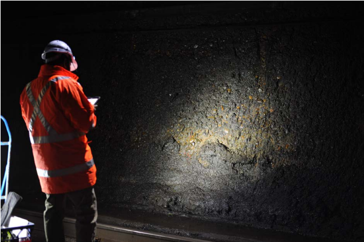
Figure 18: Water damage to tunnel lining in Tunnel 10 emphasises the locally sourced water rolled gravels that form part of the aggregate
