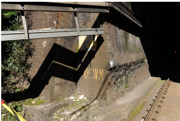
Figure 46: Detail photo of GST and existing notching, down track Sydney end portal
