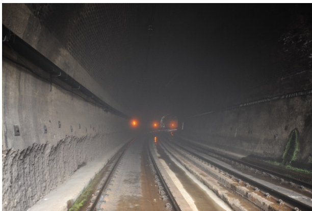
Figure 55: Internal shot of Tunnel 3 showing existing toe notching
