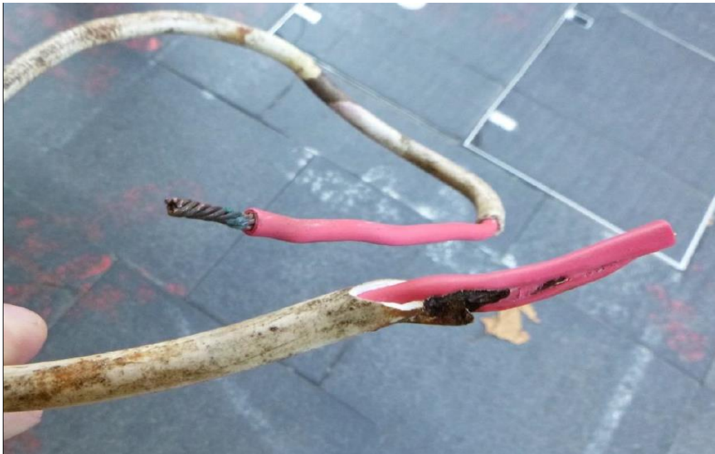
Image 2: Damaged Cable TCS 1837
