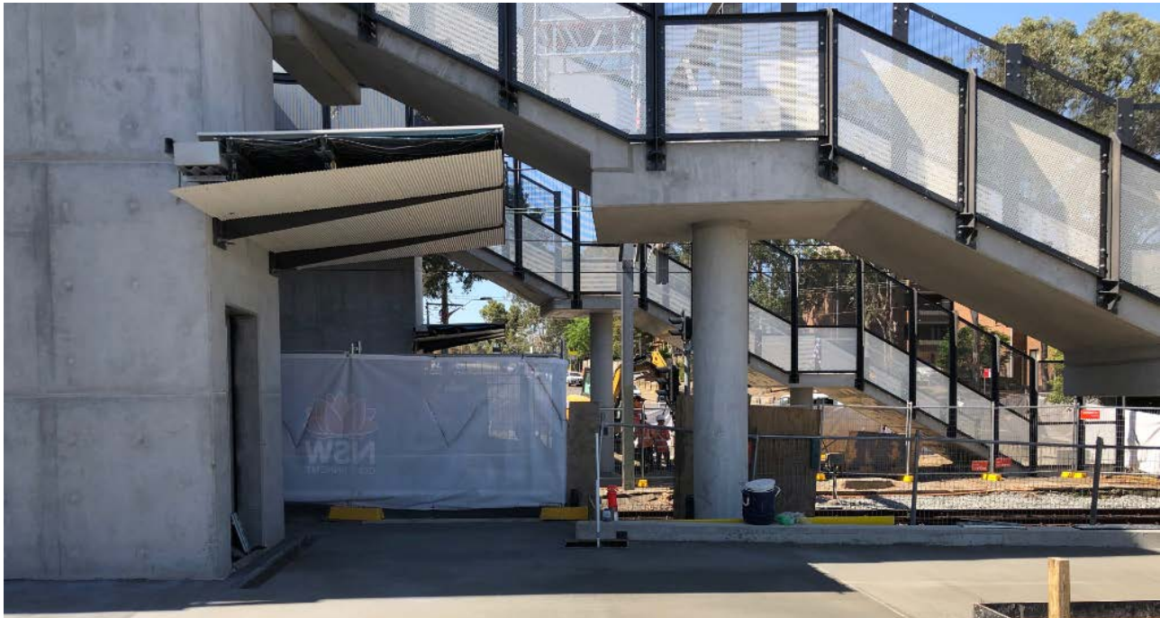
Concrete footpath and entry to new station lift and stairs at Kingswood Station
