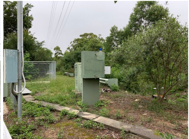
Photo 4.5 Exotic grass and forb species near the backup isolation transformer
