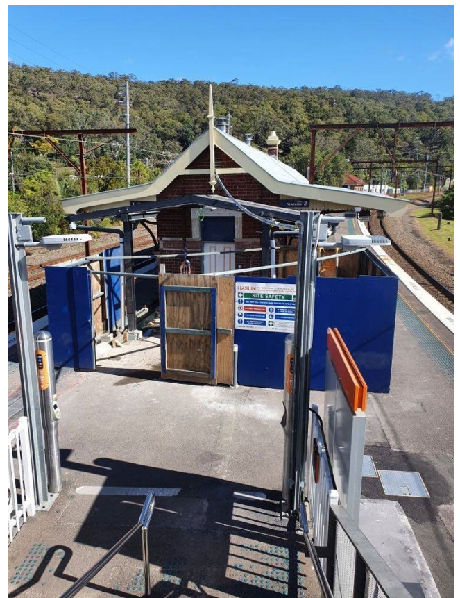
Image: The fit out of the new family accessible toilet was completed during August.
