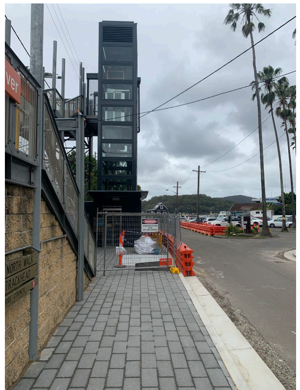
Image: Construction of new kerb and gutter and footpath to the bus stop on Dangar Road will be completed during January.
