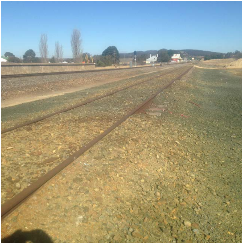
Stained Ballast on Woodlawn Siding
