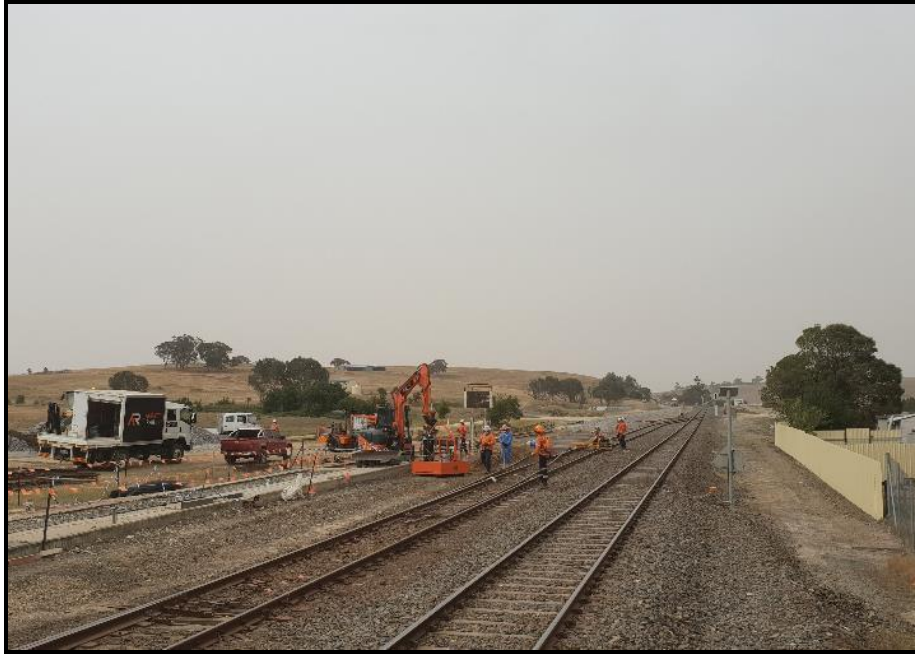
Photo 1: Tarago Rail Corridor facing north. A concrete pad remaining from the historic ore concentrate load out visible on the LHS. The Station Masters Cottage is visible on the RHS (with sheet metal fence).
