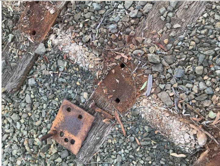
Woodlawn Siding: top pictures showing residue left behind from track cutting
