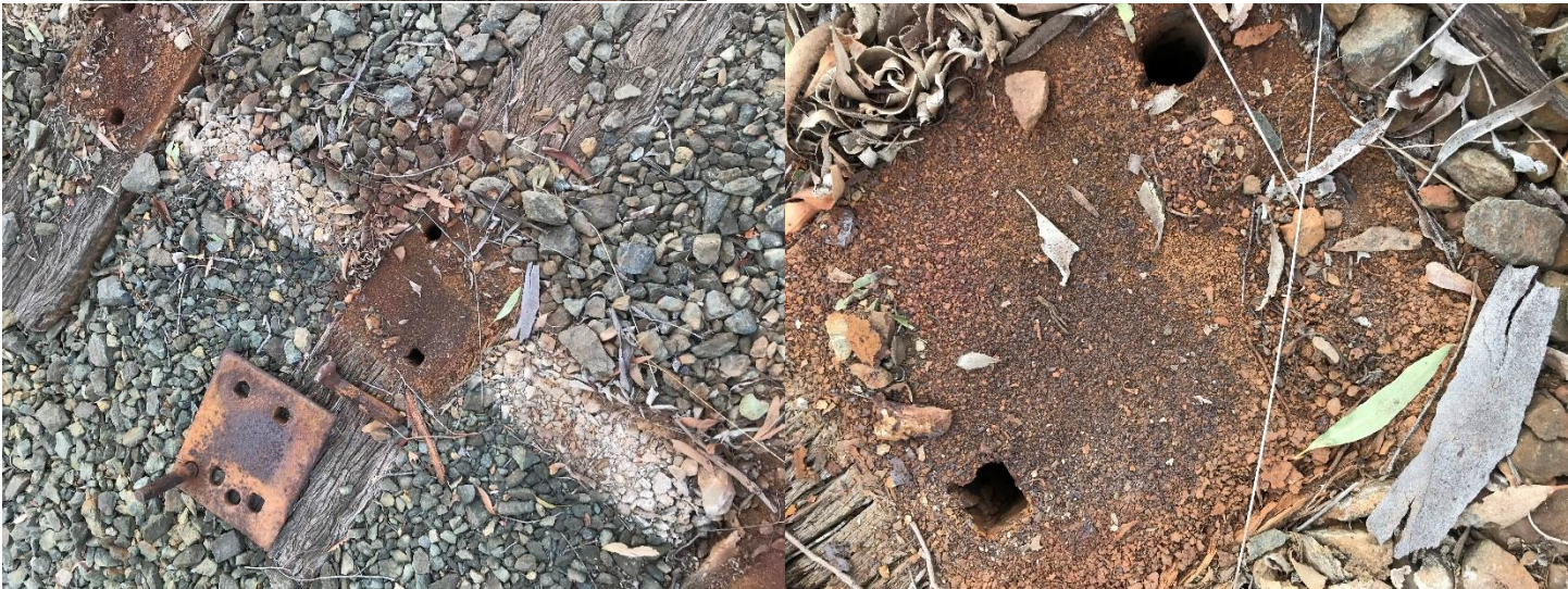
Woodlawn Siding showing degraded track work
