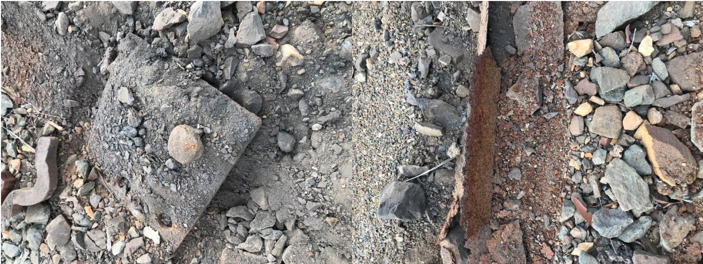
Woodlawn Siding showing fouled ballast
