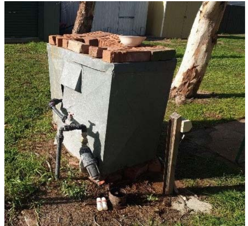
Groundwater bore at Tarago Public School
