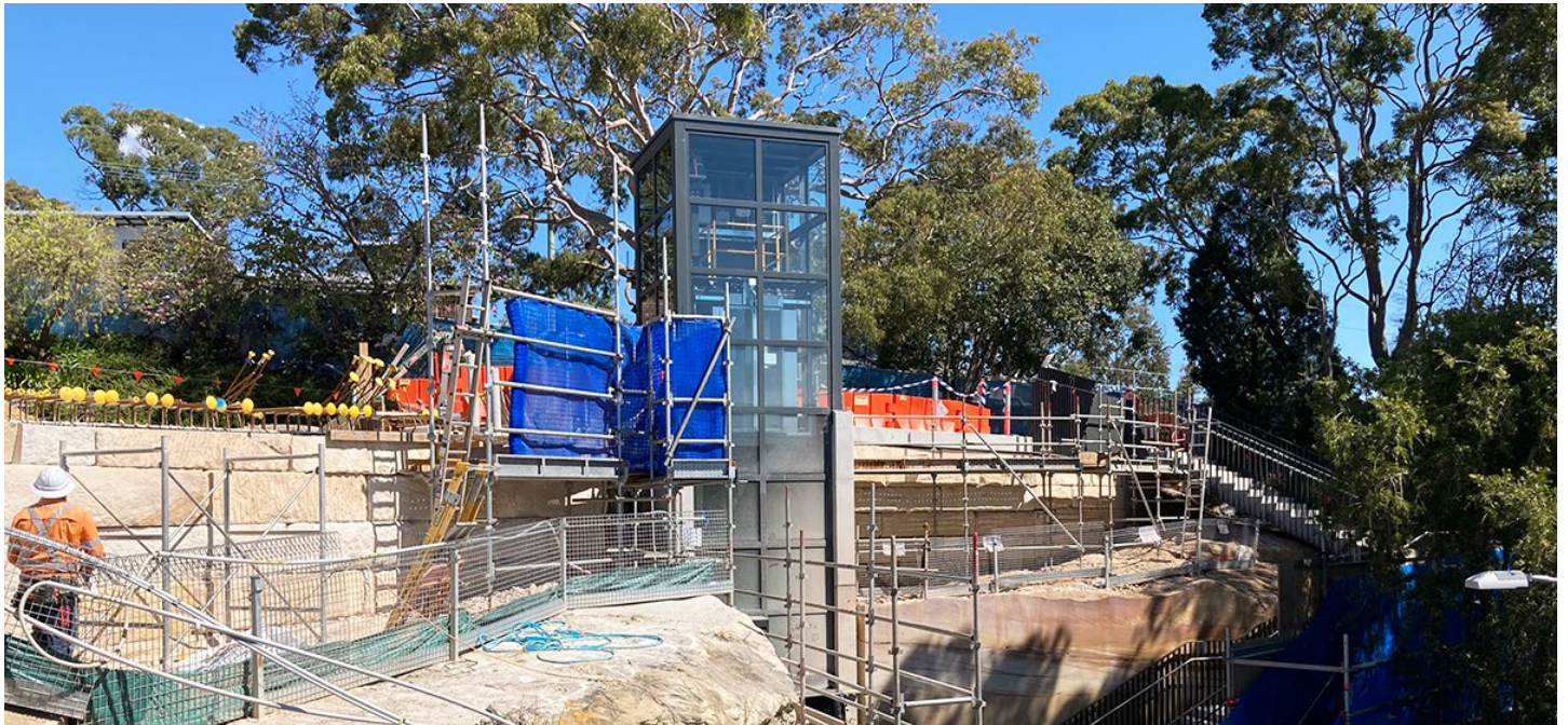
Lift and stairs from Como Parade into the station is almost complete.
