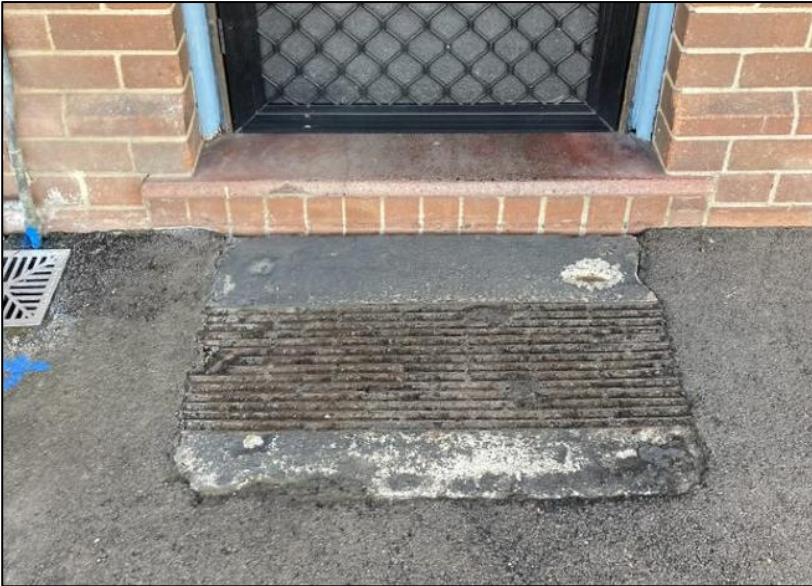
Photo 4.8 Boot cleaning grill at the entrance to Station Building C
