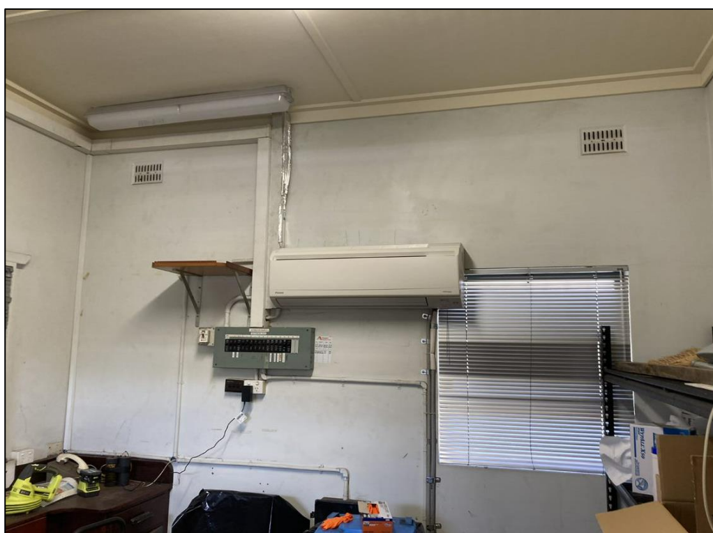
Photo 4.19 Station Building A, with cables and air-condition fixed to the south wall
