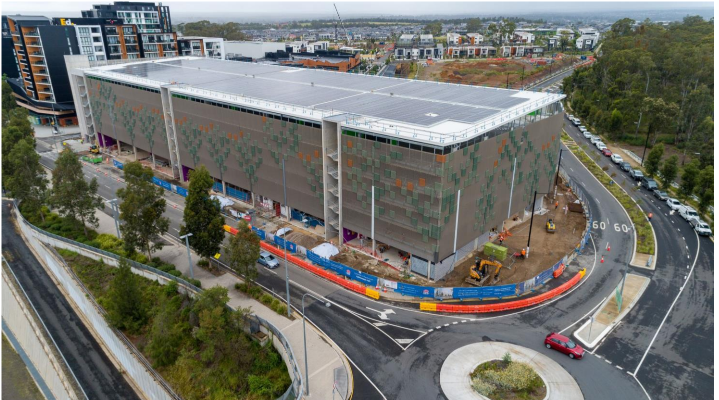
Construction progress on the new multi-storey commuter car park at Edmondson Park
