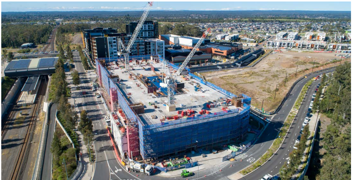
Construction progress on the new multi-storey car park at Edmondson Park, May 2021
