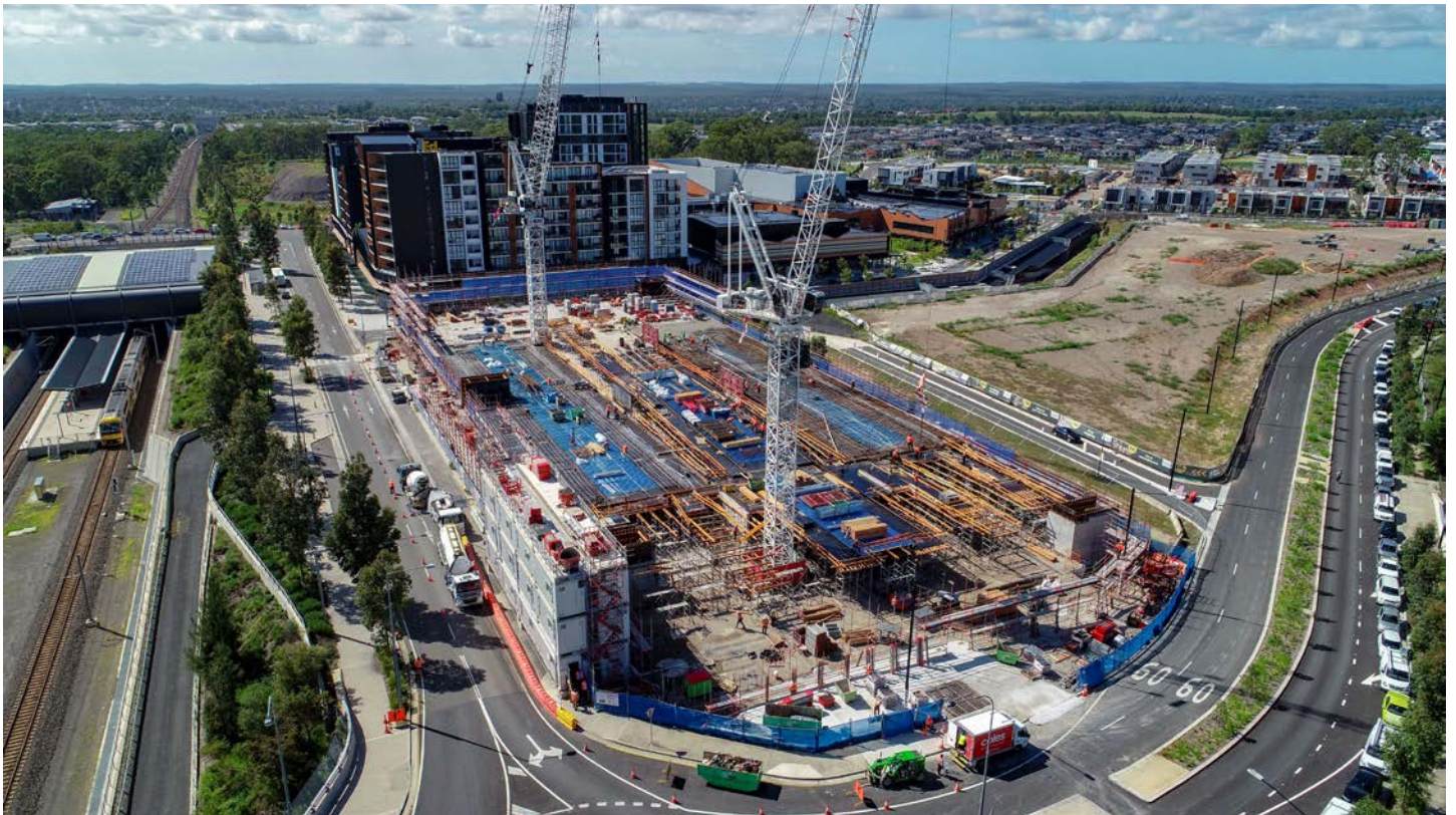
Construction progress on the new multi-storey car park at Edmondson Park, February 2021
