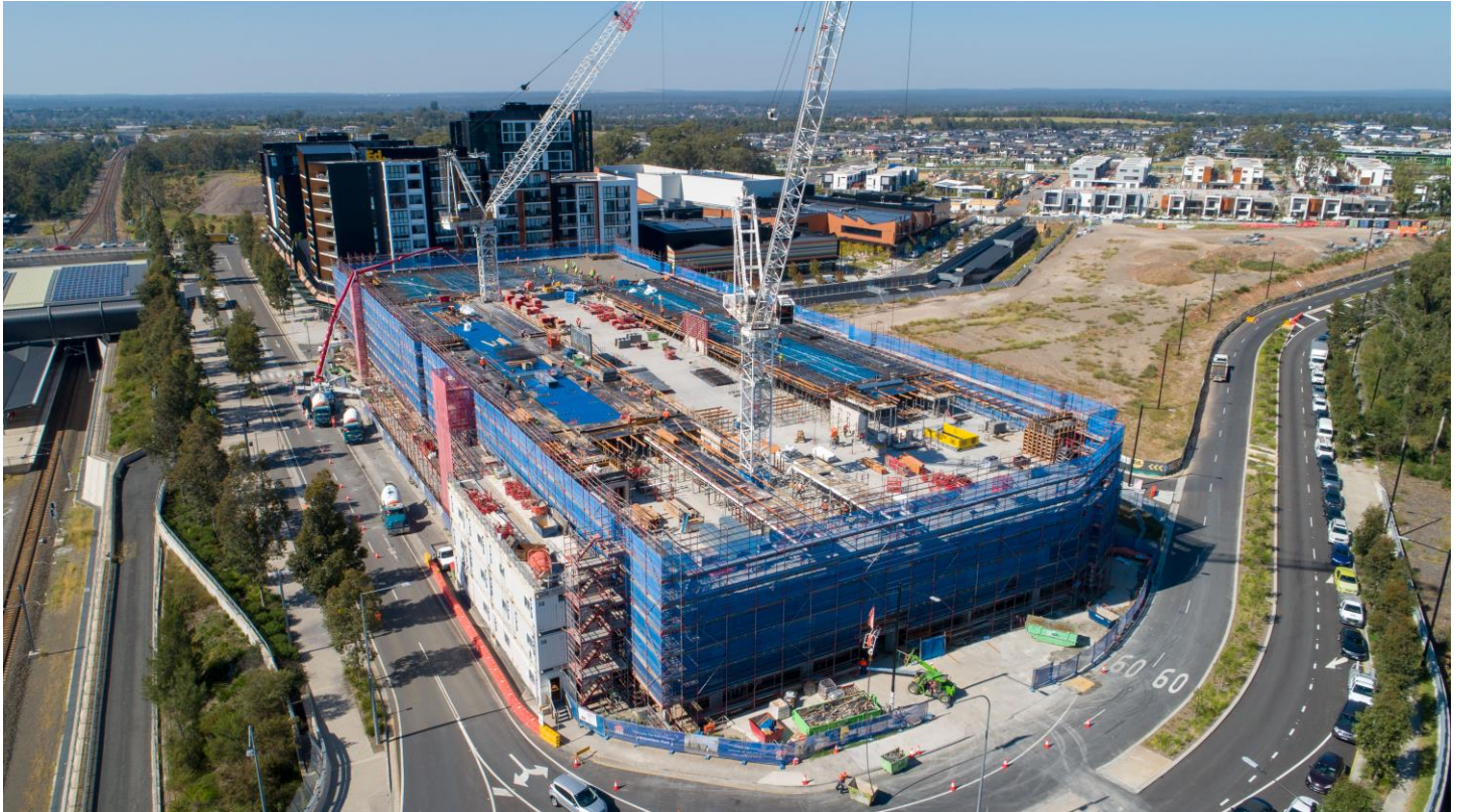
Construction progress on the new multi-storey car park at Edmondson Park, April 2021
