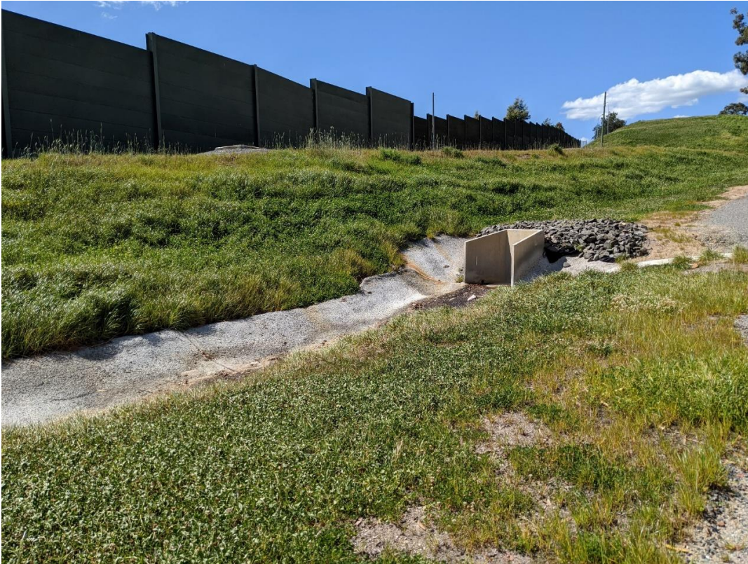
Figure 6-18 View looking north-east of existing stormwater culvert infrastructure and overland flow path on the site (Source: Advisian, 2020).
