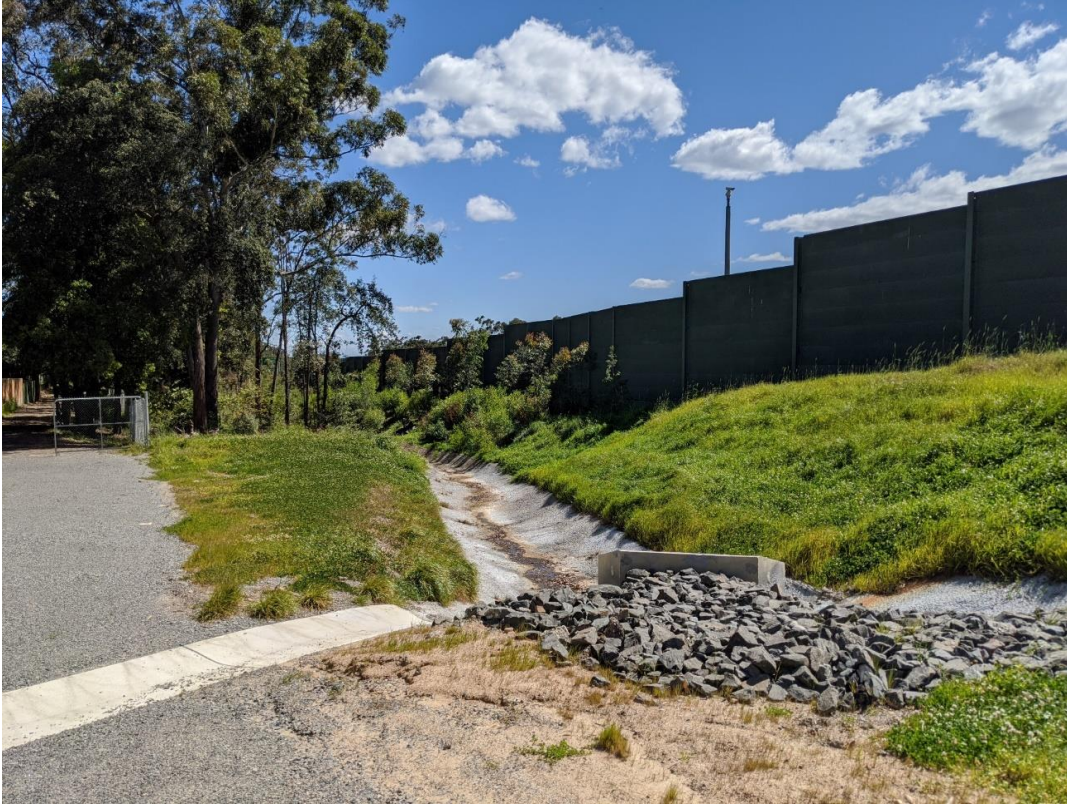
Figure 6-19 View looking west of existing stormwater culvert infrastructure and overland flow path on the site (Source: Advisian, 2020).
