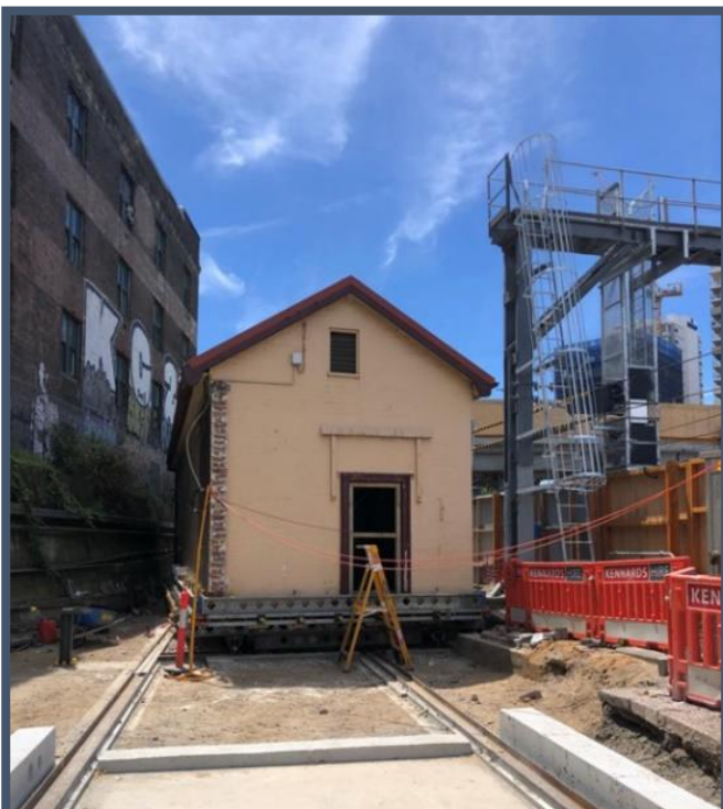
Heritage building on top of metal pulling frame after the building had been dismantled from its previous footings brick by brick. This image shows the building being rotated to move into its new position.
