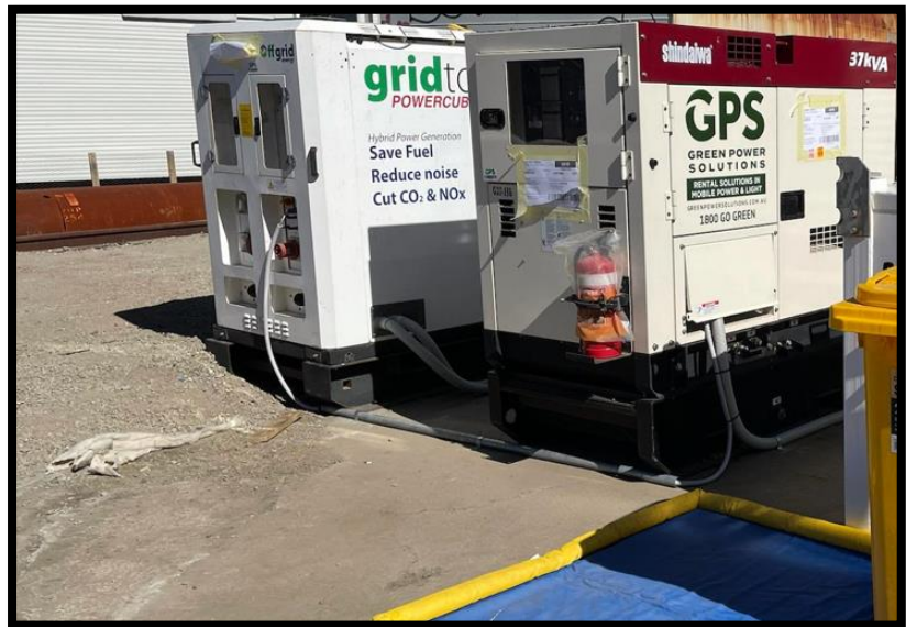
The newly installed biodiesel generator powering the project's site office.
