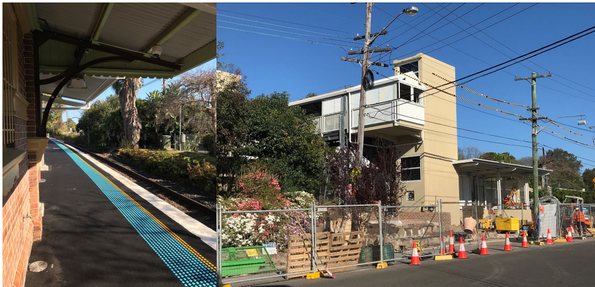
Roseville Station, September 2021 – New tactiles on Platform 2, new lift shaft and canopy on Hill Street
