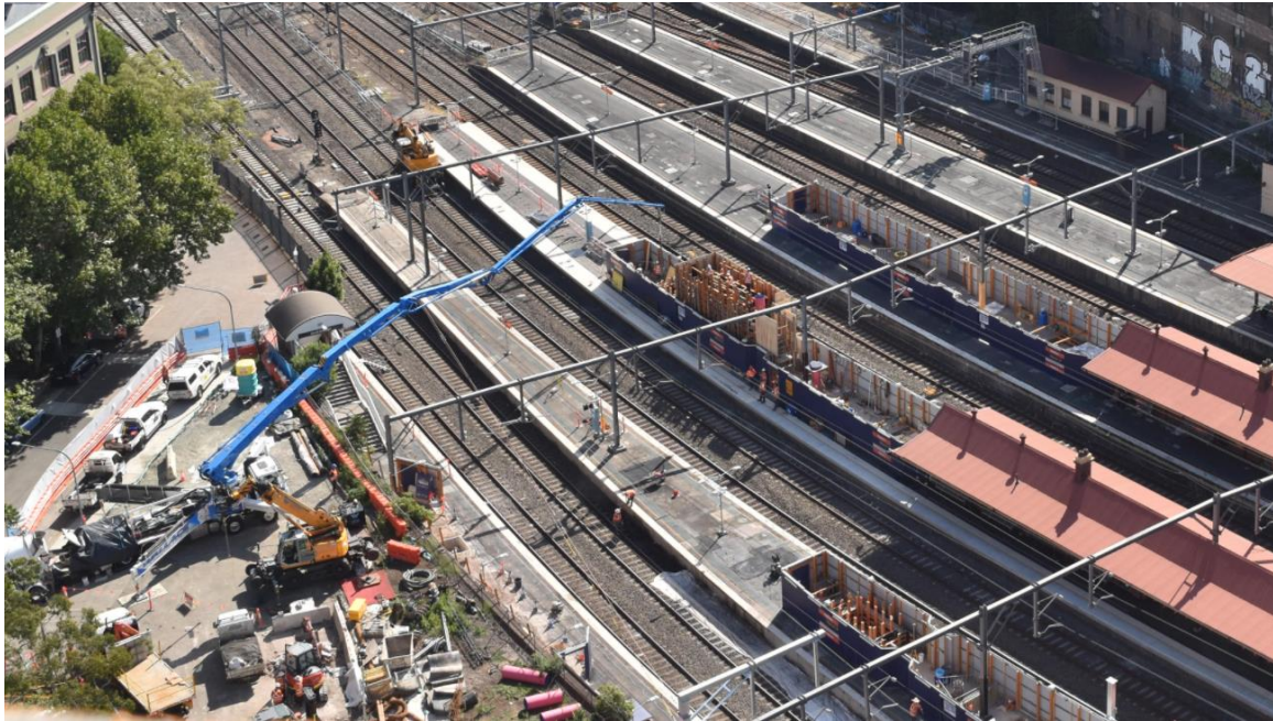
Concrete pouring on Platform 6/7 via the blue boom pump located in the Marian Street site compound. Captured in early March, this demonstrates the progress of the work on the footbridge support structures.
