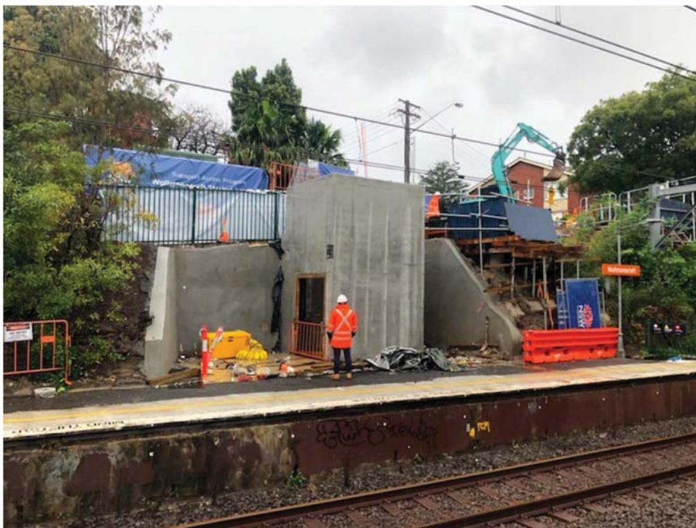
Image: construction of the lift to Platform 1 during the March 2021 weekend work
