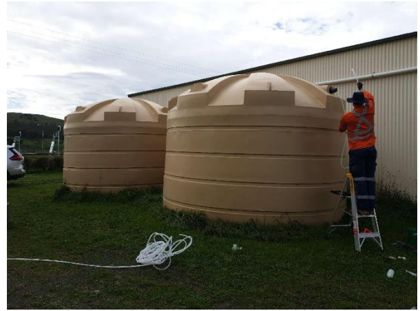
Photo 26 Water tanks at the Tarago RFS. Date: 25/03/20
