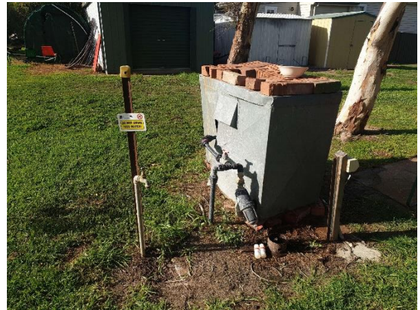
Photo 30 Tarago Public School underground bore. Date: 24/03/20
