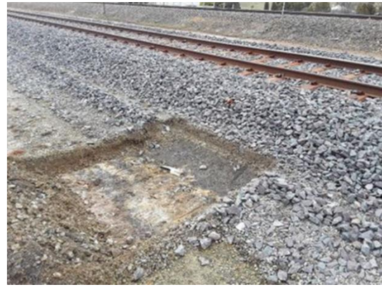
Photograph 38: Composite sample RRE_TP02 collected from shallow test pit adjacent the northern portion of the rail formation. Sample collected 19 August 2020.
