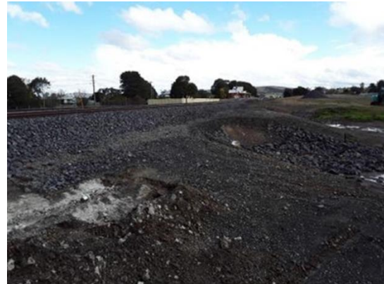
Photograph 42: Composite sample RRE_TP06 collected from shallow test pit adjacent the rail formation. Sample collected 19 August 2020.
