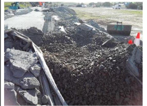
Photograph 47: Composite sample RRE_SP01 collected from the southern face of onsite stockpile comprising fouled ballast impacted by ore concentrate. Sample collected 19 August 2020.
