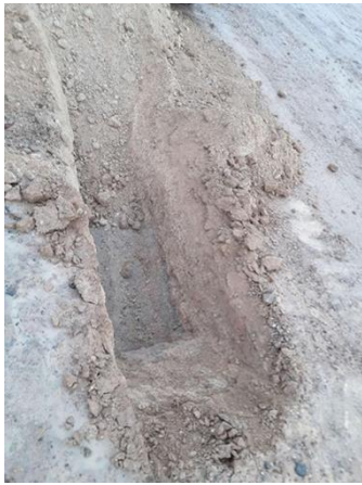
Photograph 33: Test pit LO_TP04 terminated at 0.8 mbgl due to refusal on concrete slab.
