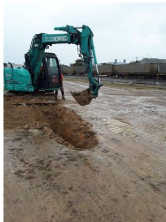
Photograph 30: Test pit LO_TP03 located within the footprint of the former Loadout Facility . Sampled 19 August 2020.
