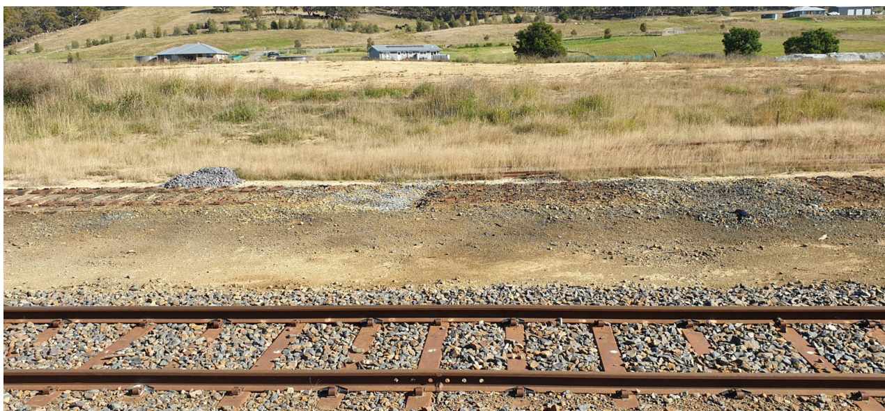
Photograph 1: Polymer Sealant on the Woodlawn Siding in January 2021
