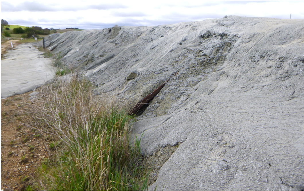
Photo 5: Stabilised sand applied as stockpile capping (western side of stockpile). Metal sleepers used as weights during initial placement of geofabric marker layer remain partially visible.
