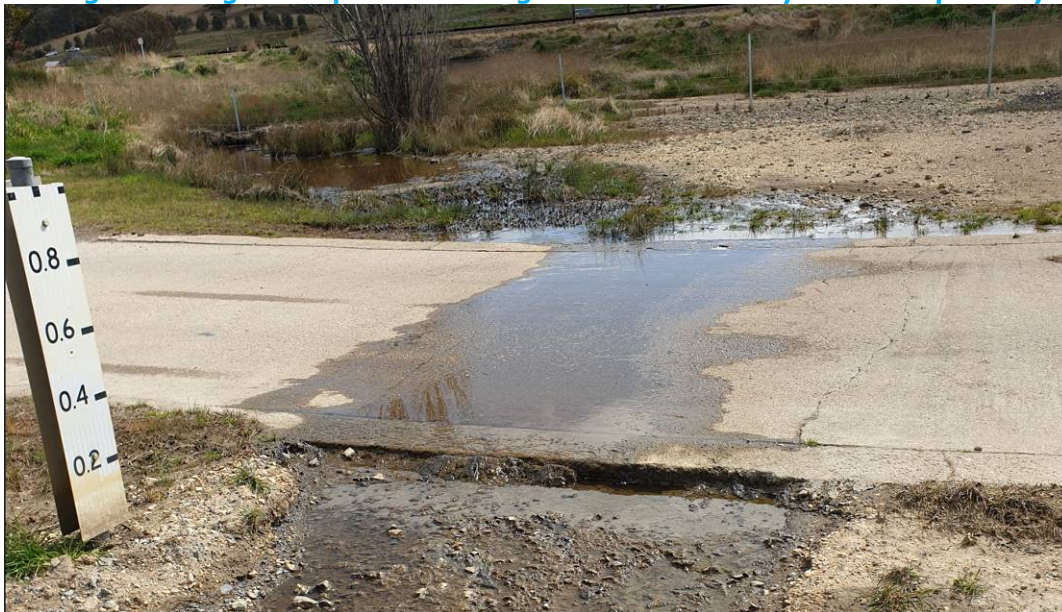
Photo 6: Surface water discharging across Boyd Street downstream of the middle culvert was visibly clear.
