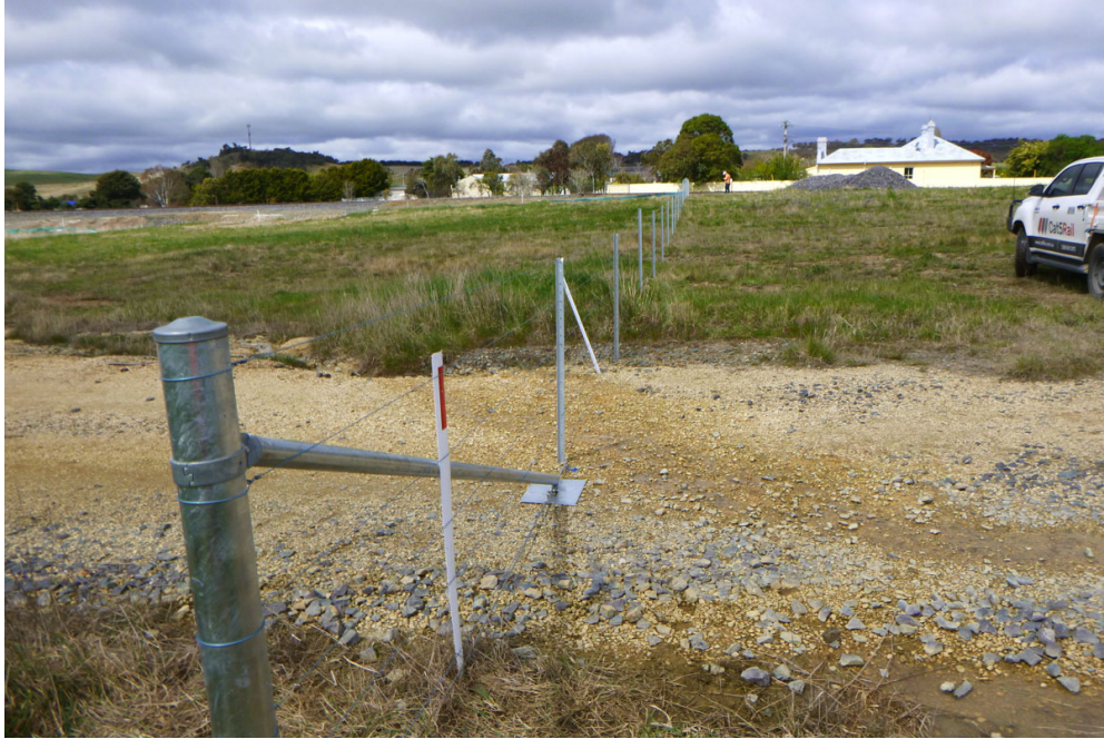
Photo 1: Fencing to limit vehicular access to the northern portion of the Tarago Rail Yard including upstream of the middle and northern culverts. 106 Goulburn Street visible in the background provides a reference point.
