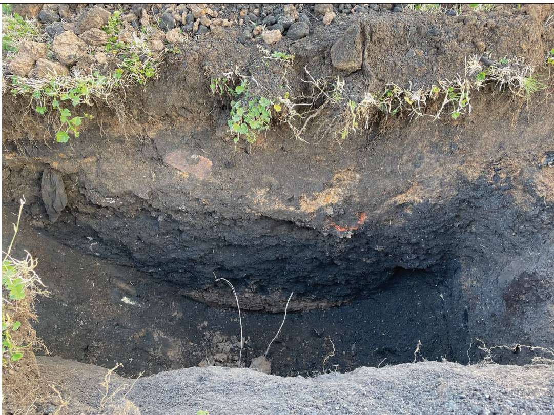
Photograph 18 Ash fill material overlying natural sandy clay material observed during the advancement of TP27.
