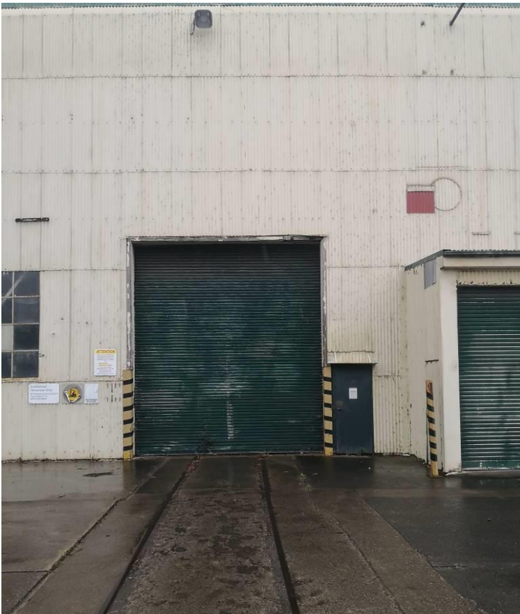
Figure 14 Part of the East elevation with significant embedded track. Tracks to be retained and doors to be replaced for rolling stock access. The extension from the late 1980s over the northern door is to be removed to return the elevation to the original alignment.
