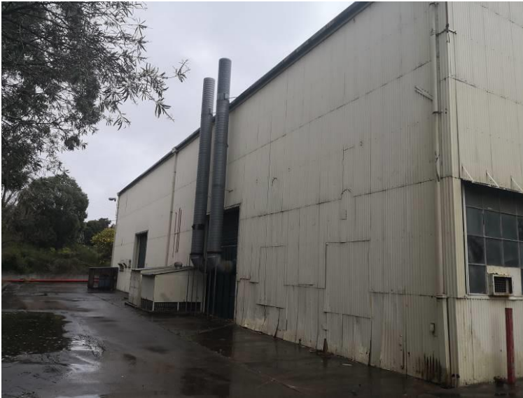
Figure 7 View of the West Elevation. The elevation is a patchwork of alterations and minor additions completed from the 1950s with the introduction of diesel electric maintenance tasks. The bottom level of the sheeting has suffered from collision damage and rust in contact with the slab surrounds.
