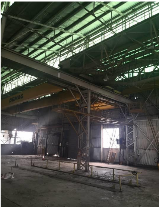
View of the interior including the original Crane LC591
