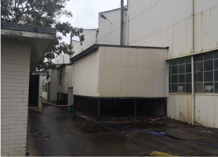
Figure 9 View of the skillion roofed extensions to the Tank Annex. These timber framed structures were built with wire screened open bases to accommodate diesel electric maintenance works introduced in the late 1950s. The timber frames have rotted and the structures are not capable of certification. It is proposed that these be removed to accommodate the access.
