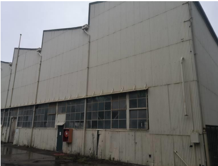
Figure 8 View of the western end of the North elevation. The original galvanised iron sheet cladding and steel framed windows are generally intact and retain their significance. The rain heads have been replaced. The bottom level of the sheeting has suffered from collision damage and rust in contact with the slab surrounds. The steel framed windows are affected to various degrees by rust and have sustained damaged glass panes and many replacement panes.
