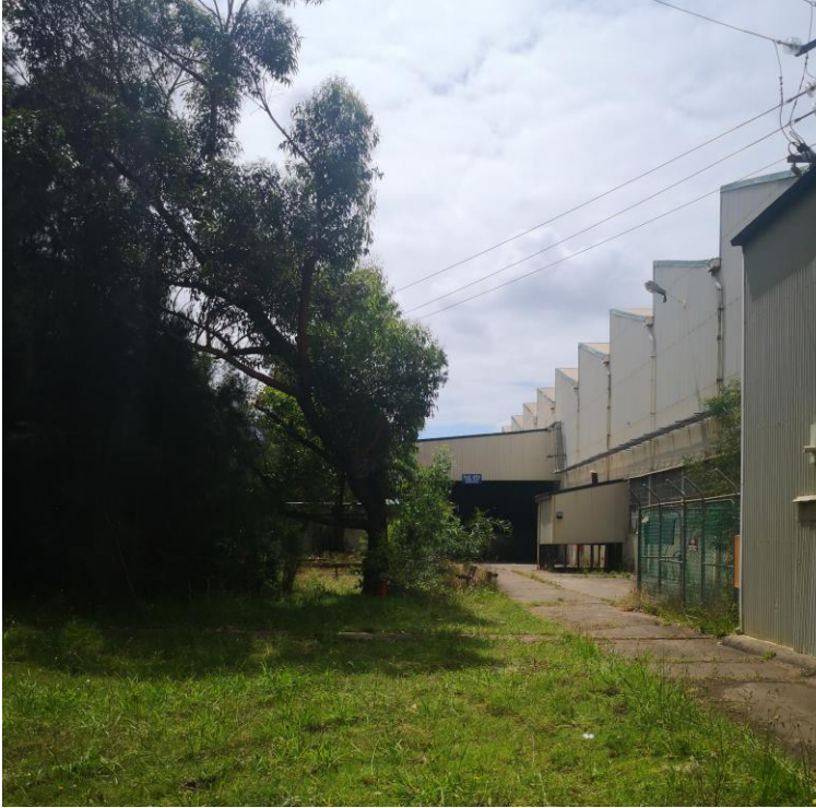
Figure 11 View of the second tree in the vicinity of the shed. This tree is in poor condition and is to be removed for the required access road and for improved clearance to the main Electricity supply cabling overhead. The tree has been severely and unevenly pruned on several occasions to provide clearance for the main electrical overhead line entry to the building.
