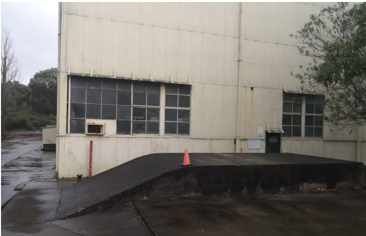
Figure 6 The significant tank ramp at the South west corner. Areas of the window band have sustained various alterations including removal for doors and air-conditioners. Some areas have simply been sheeted over.
