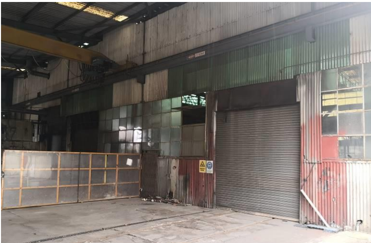
Figure 12 View of the eastern end of the North elevation within the open skillion extension. The alterations and addition of the large skillion extension were part of changes in the 1980s to accommodate the Electrical Maintenance Centre. The damaged walls and windows are to be restored to conserve and secure the building envelope.
