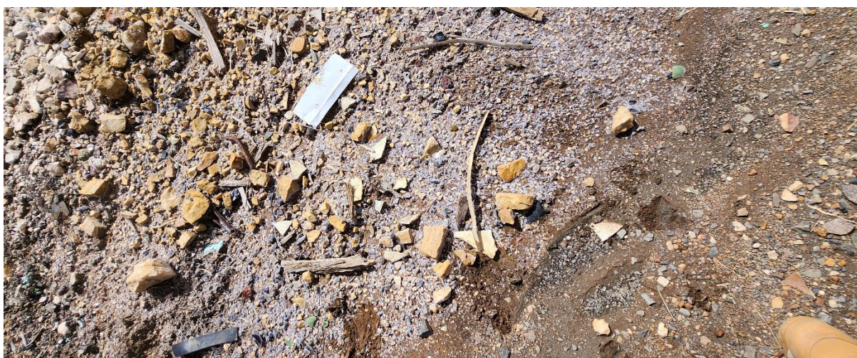
Plate 8. Wheat yard siding bonded asbestos fragments
