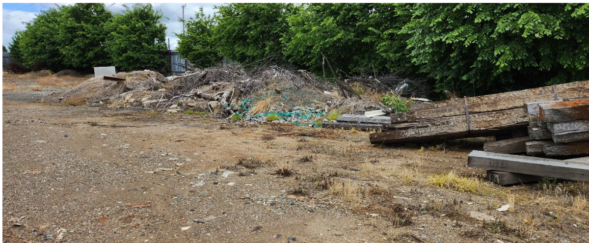
Plate 3. Waste and timber stockpiles
