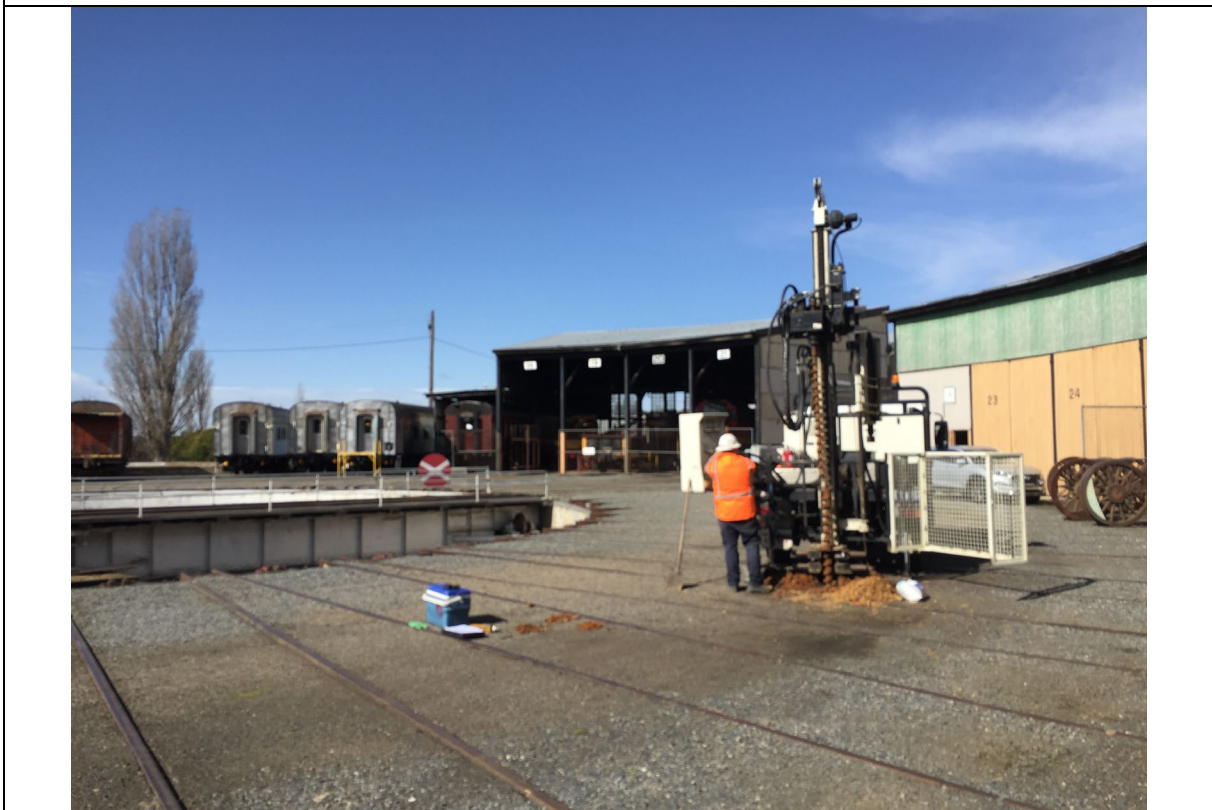
Photograph 20 View south during the advancement of borehole BH07, to the east of the Engine Shed within the Roundhouse.
