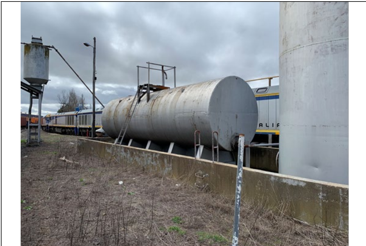
Photograph 5 View north towards the decommissioned diesel aboveground storage tanks.
