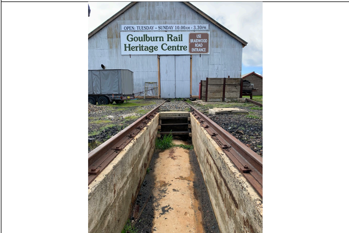
Photograph 10 View north towards the maintenance pit (foreground) and former workshop / machine shop in the background.
