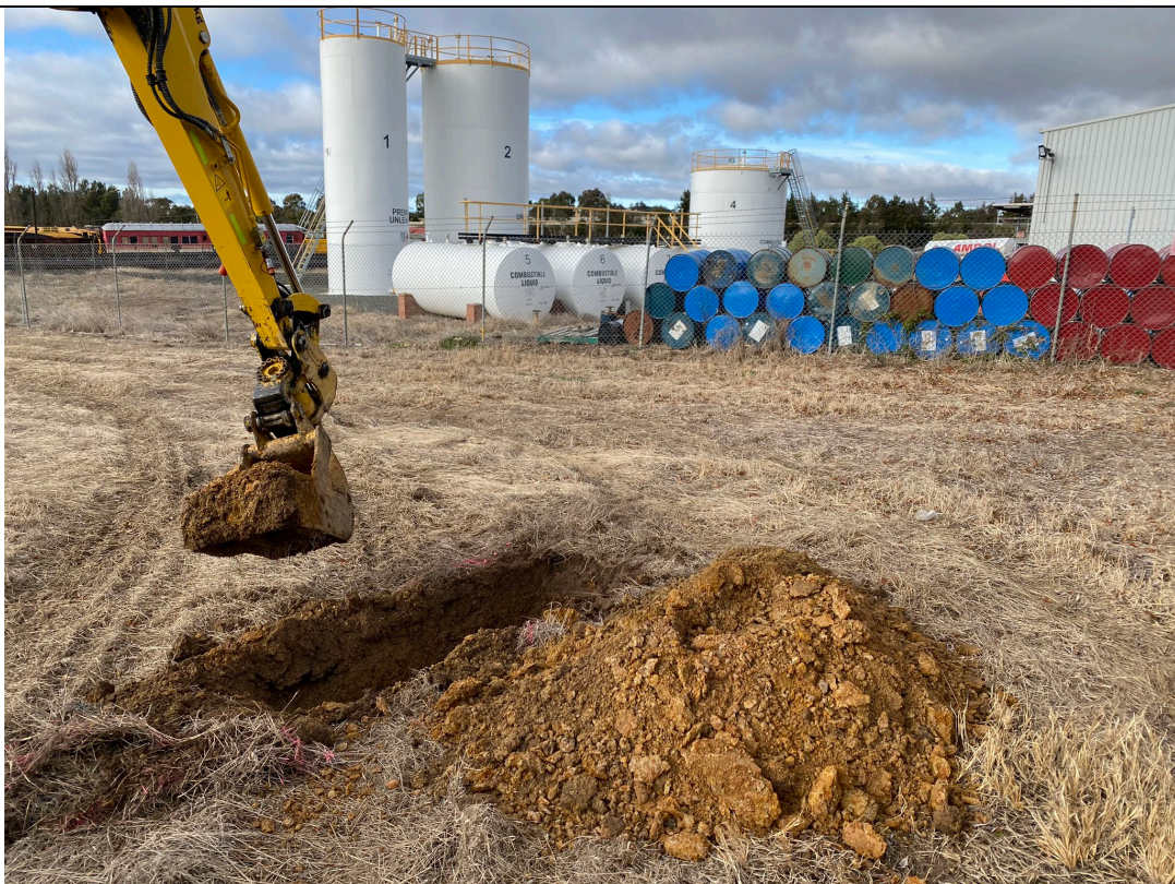
Photograph 22 View south towards the operational Caltec Fuel Depot. Natural material identified within Area C, within test pit TPC14.
