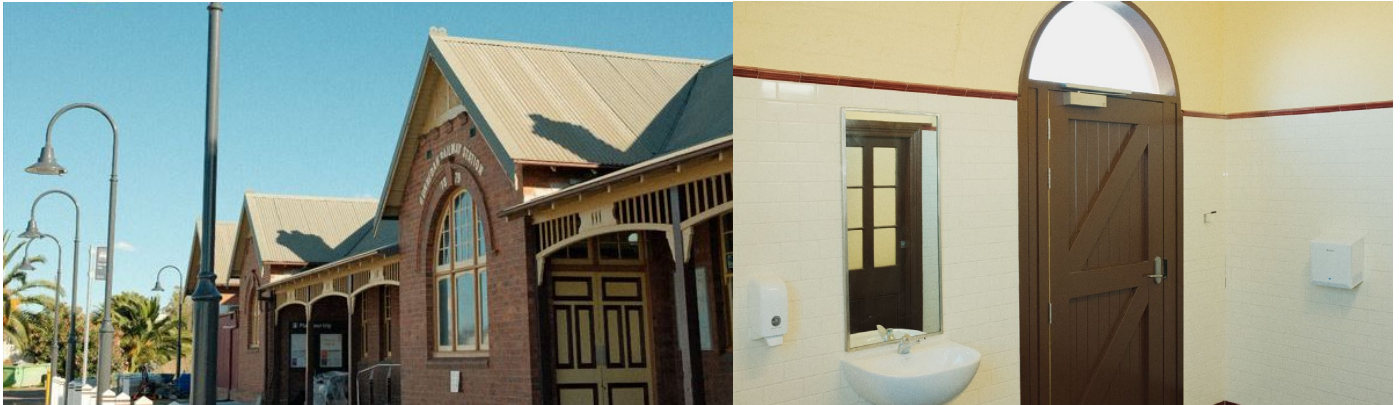
Pictured from left: Restored waiting room, Toilet entrance in original heritage configuration
