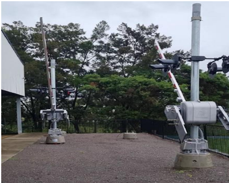
Figure 24: Boom gates in operation during the Self-Contained Cost-Effective Level Crossing Solution Project trial, Stage 1.
