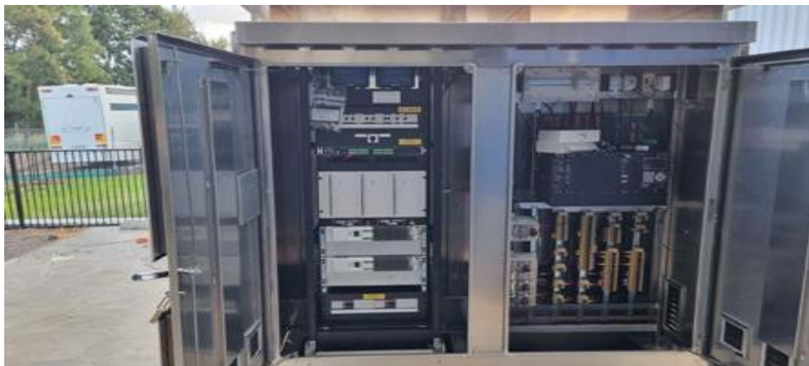
Figure 23: Solar powered location case interna (sentinel power rack on left. GCP on right.)
