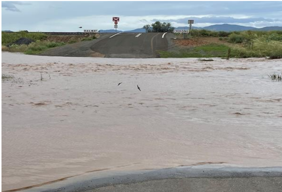
Figure 1: Floodwater at the ARTC constructed Bulunbulun Road, Breeza level crossing
