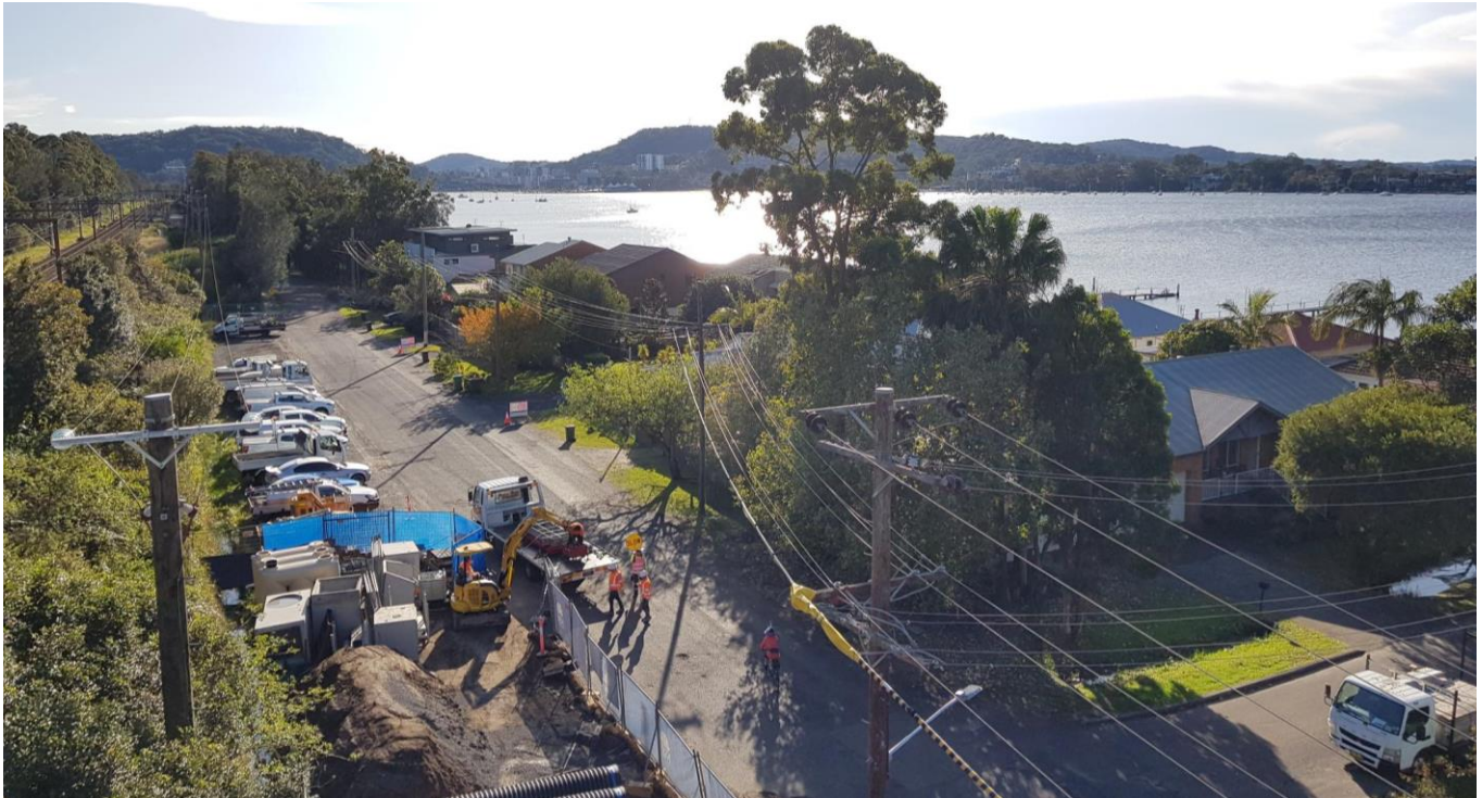
View from the top of the lift shaft on the Kurrawa Avenue side of Point Clare Station, July 2022
