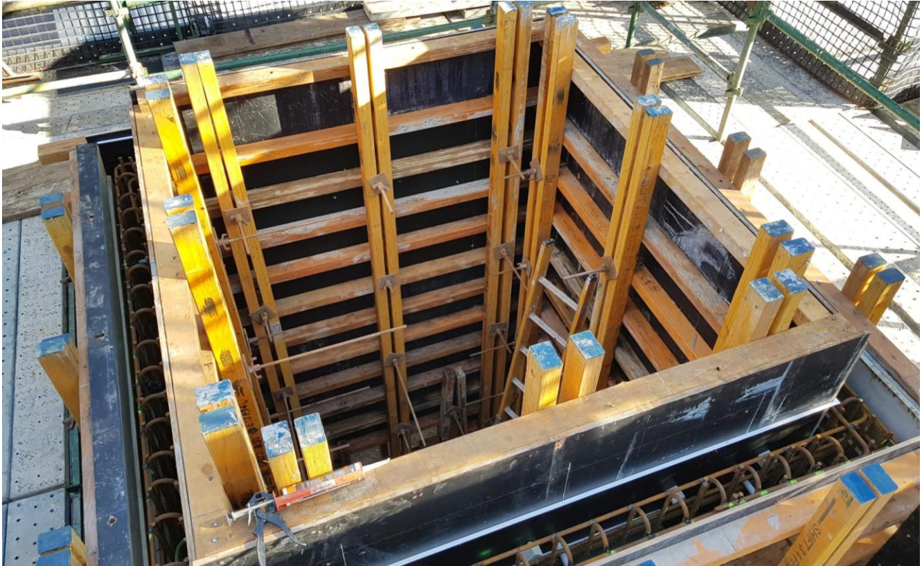
Lift shaft formwork ready for concrete pour on the Kurrawa Avenue side of Point Clare Station, July 2022
