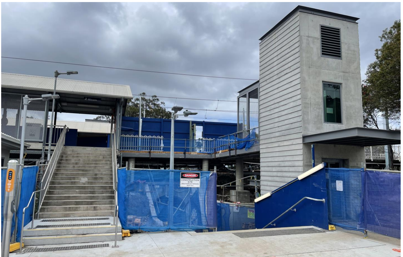
Pictured: New station entry on Brisbane Water Drive with lift construction nearing completion.
